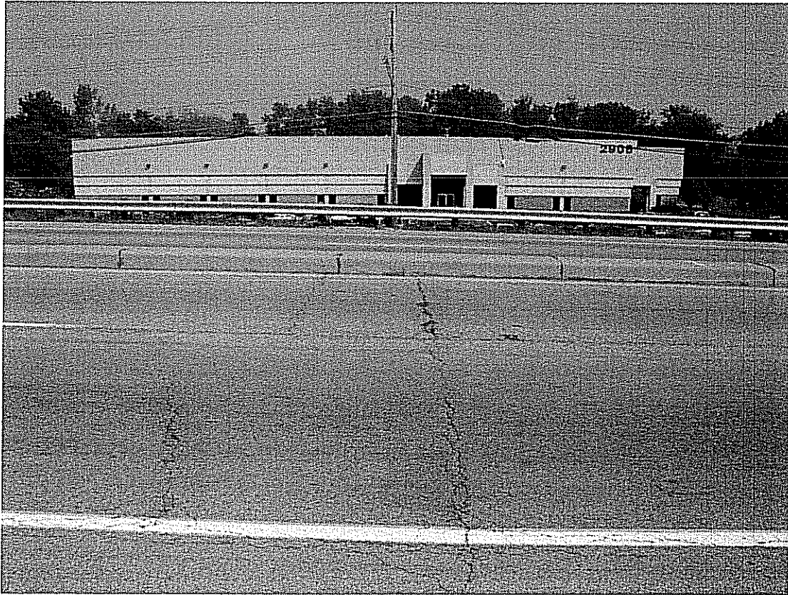
Concrete Joint reflective cracking (typical throughout project)
