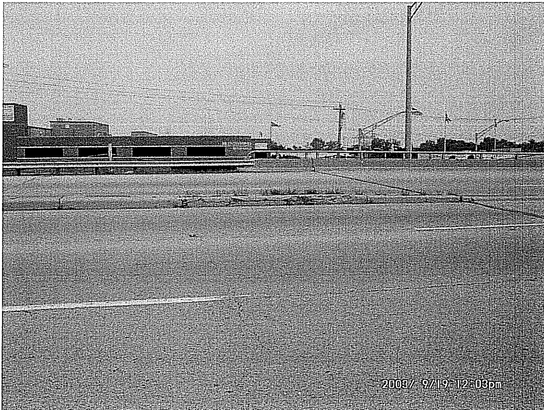
Concrete Median deterioration at Medallion Drive overpass
