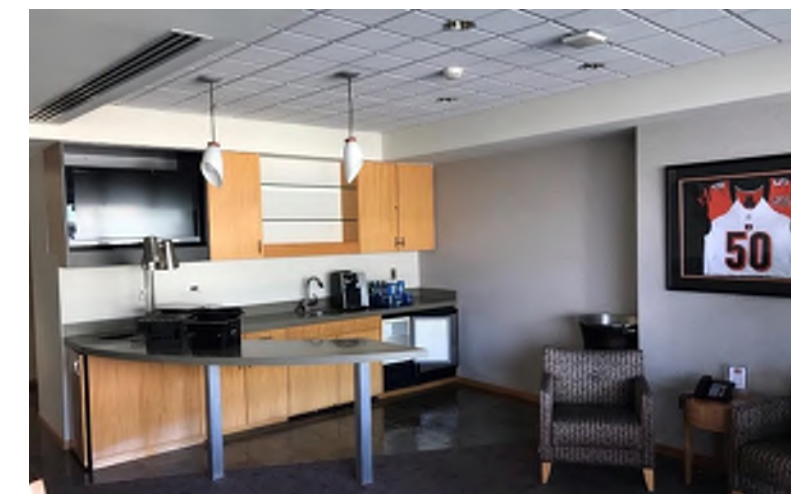
Access point on the suite ceiling grid
