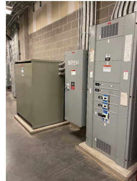
Typical emergency transformer, ATS, and distribution panel
