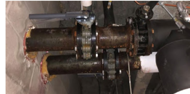
Exposed pipe and valve flanges in dual temp main in mezzanine in sector 8.
