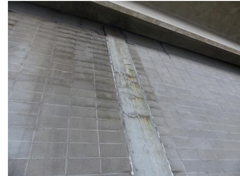
Delaminated concrete on column along exterior concrete masonry wall at service level
