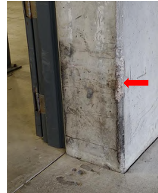
Exterior ramps – damaged wall corner
