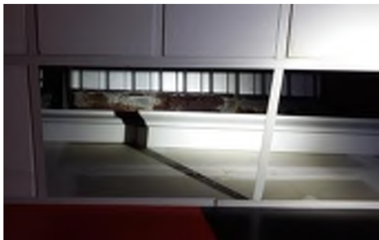
Deteriorated gutter at end of subroof
