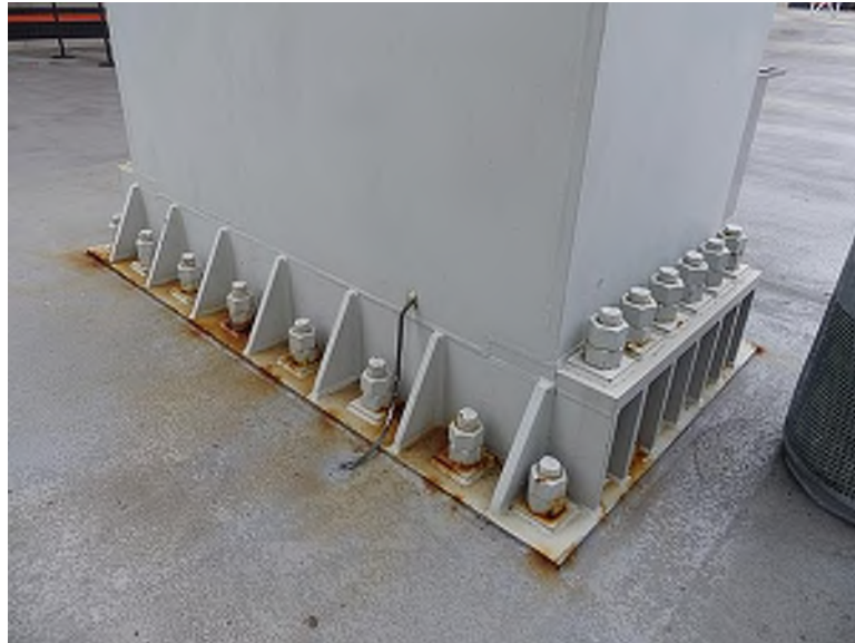
Corrosion along the baseplate of the south scoreboard support column
