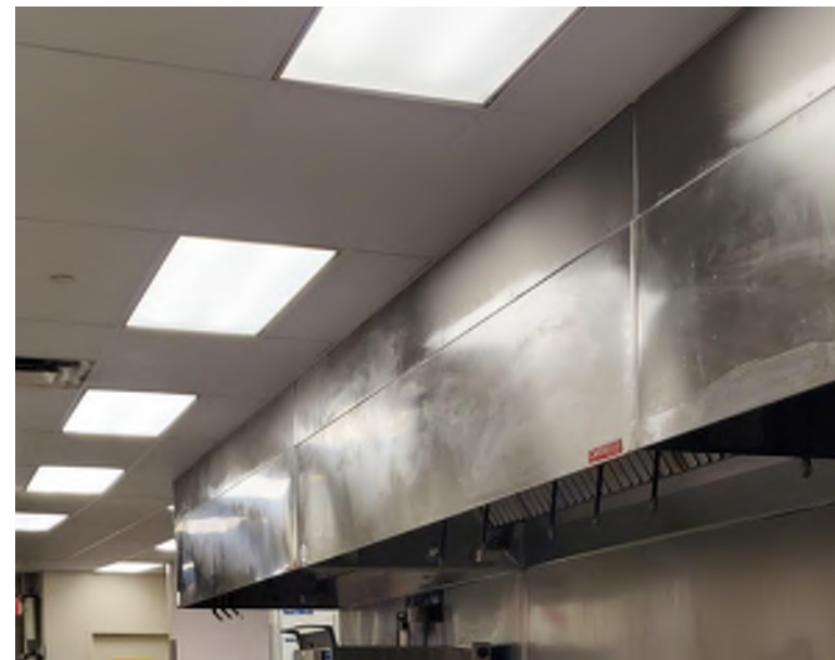
Typical kitchen lighting
