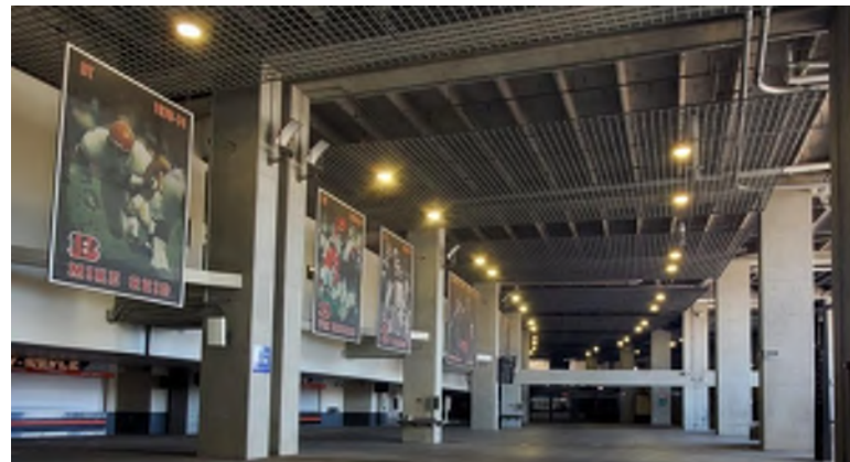
Typical LED high bay lighting
