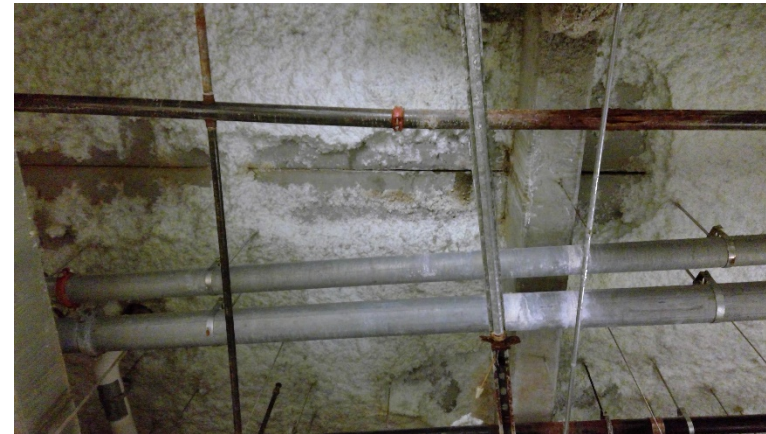
Leaking water from Plaza above in mechanical room
