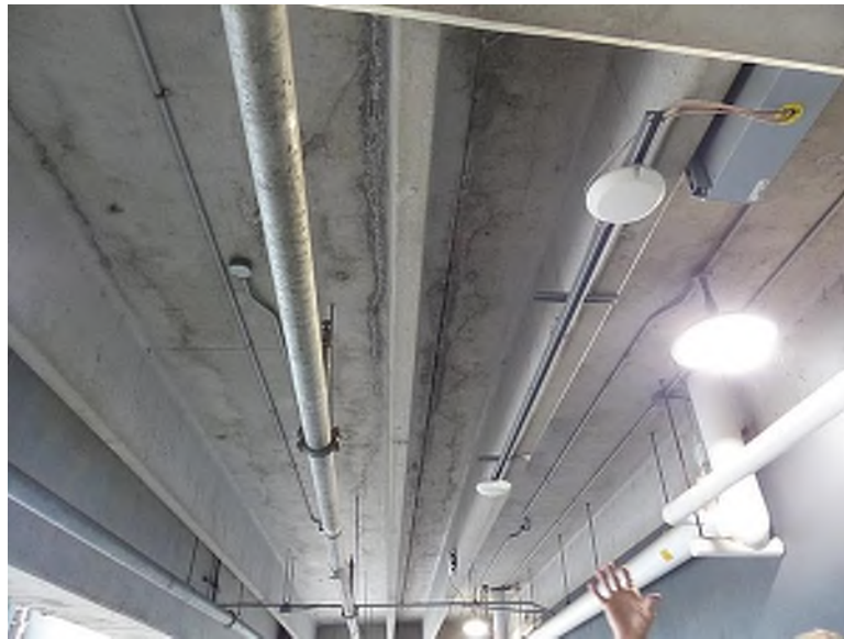
Leaching along the underside of precast double tees (Club Suites West, northwest concourse)
