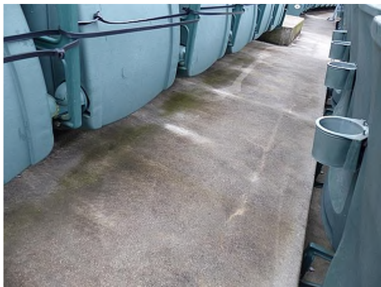
Biological growth along the top surface of precast seating risers (Club Level, Section 203 Row 3)
