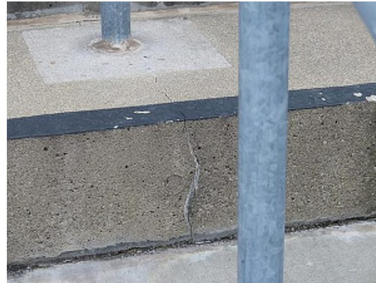
Transverse crack through the intermediate step at the location of the stanchion (Club Level, Section 211 Row 5)
