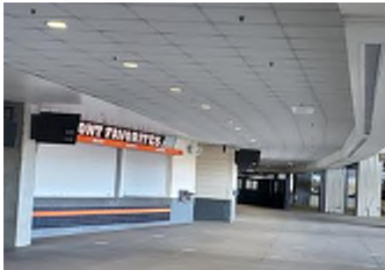
Typical concourse low ceiling downlights
