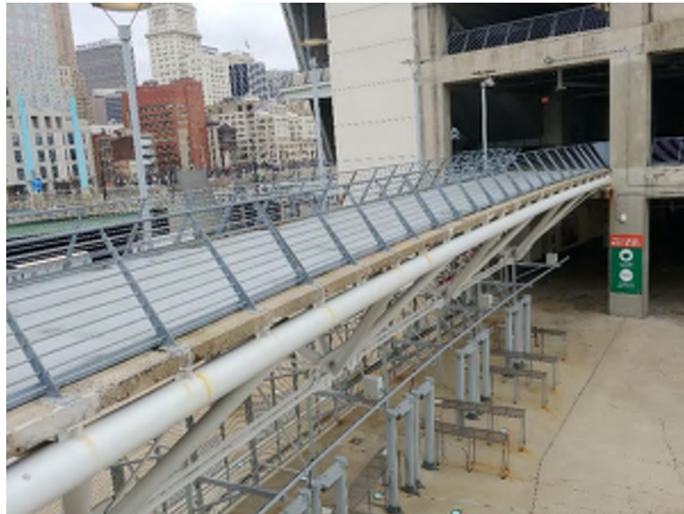
North Bridge over Gate C with water damage
