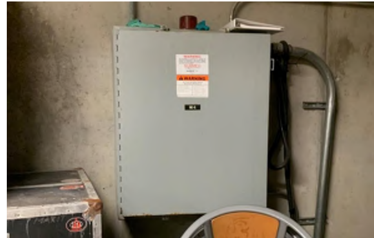
Sewage pump control panel
