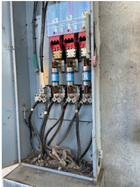
Exterior broadcast truck power panel with debris and uncovered openings
