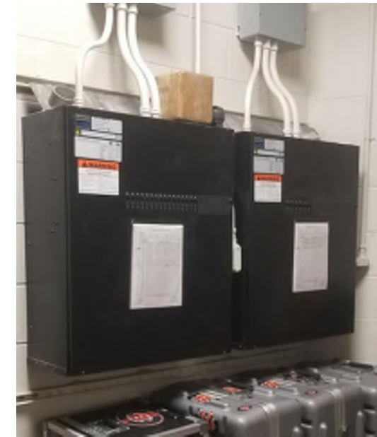
Auditorium Lutron lighting control panels
