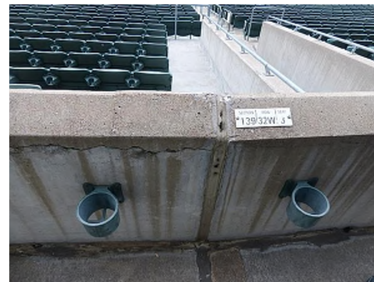
Cold joint located between the top of the precast wall panel and the sloped concrete cap (Lower Bowl, Section 139 Row 32W Seat 3)
