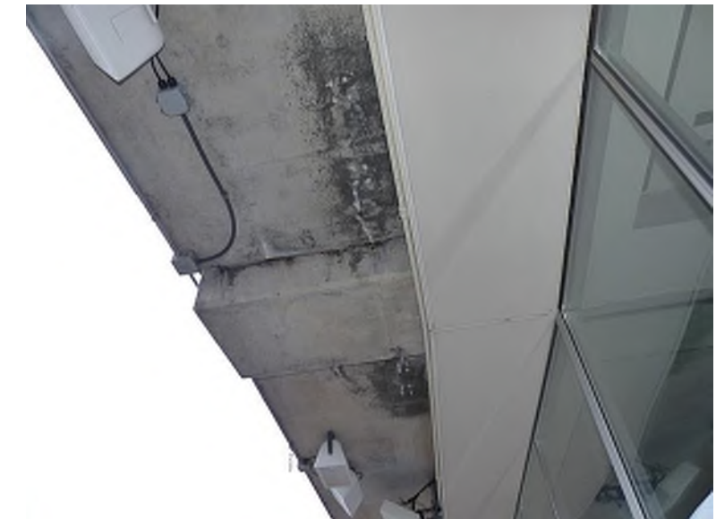
Leaching along the underside of the bottom tier of the precast concrete riser (as seen from Plaza Level, Section 140)
