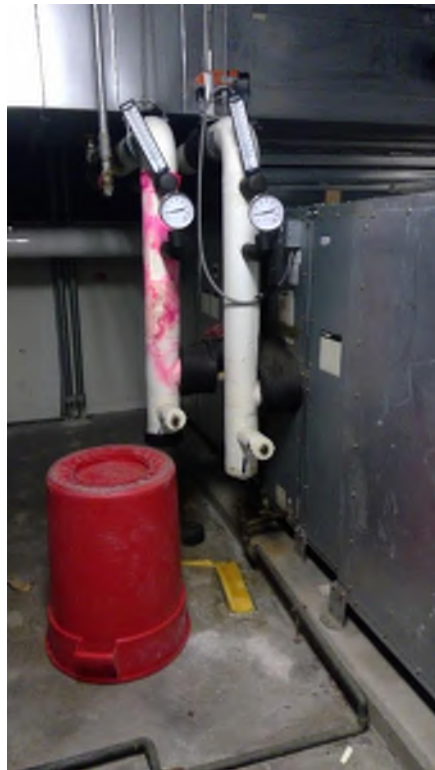
Leak in pipe riser at coil connection of AHU-UL-16
