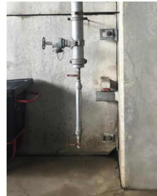
Upper ball valve should be opened on dry system drains.
