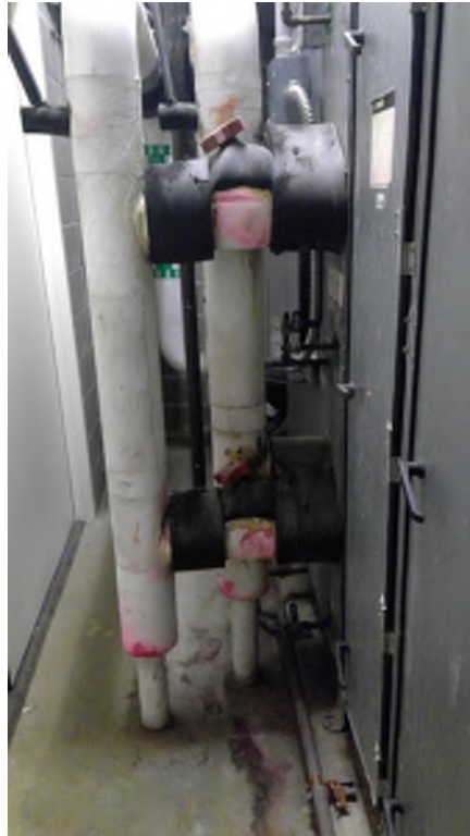
Minor insulation wear and glycol leak at coil connection of AHU-P-2
