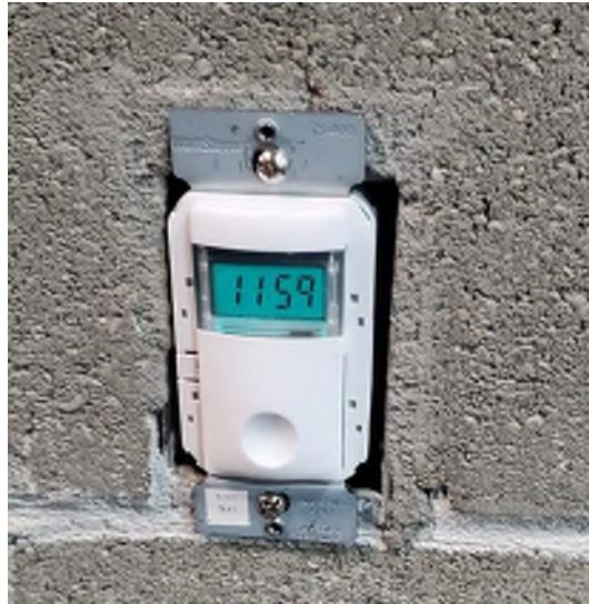
Typical lighting control timer
