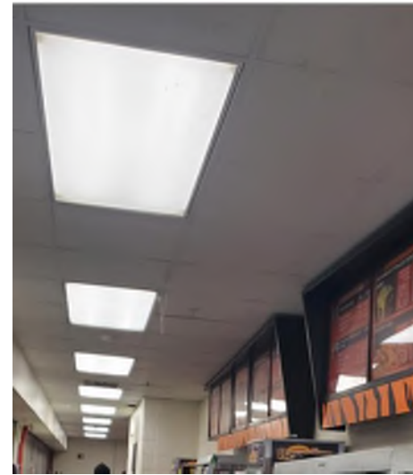
Typical concession area lighting
