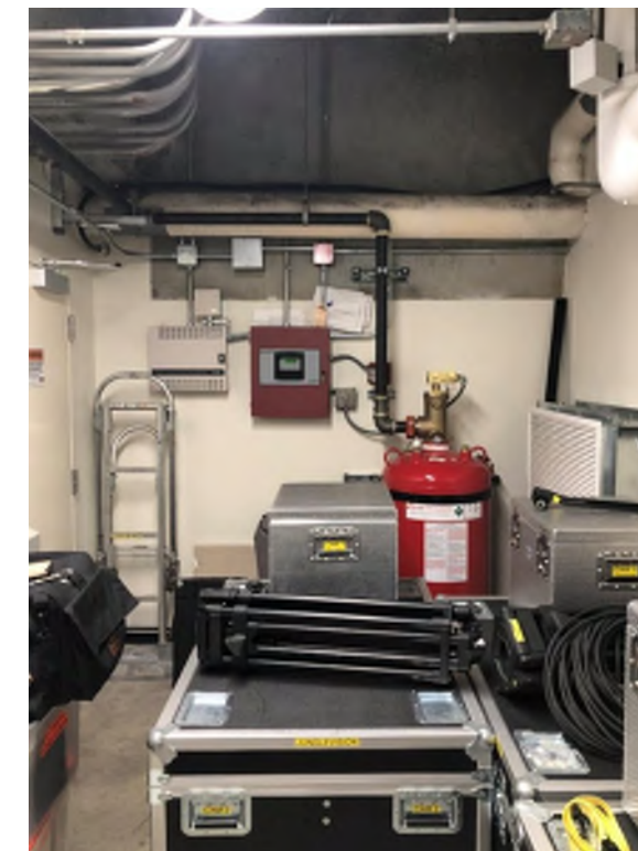
Clean Agent Storage Room Clearances
