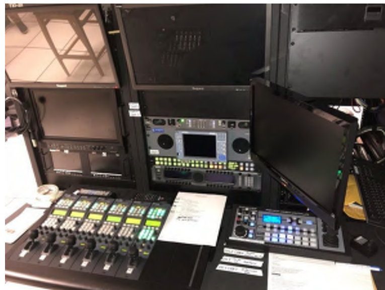
Camera control station supports (6) manned cameras
