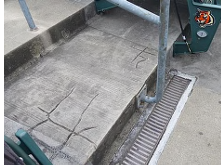
The material used to repair cracks in the precast risers has been worn away (Lower Bowl, Section 142 Row 1). Concrete coating build ups are causing water to disperse away from drains causing ponding water in the seating aisles.
