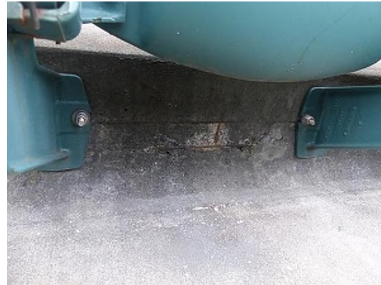
Exposed longitudinal reinforcing steel along the vertical surface of a precast seating riser (Lower Seating Bowl, Section 140, back rows)
