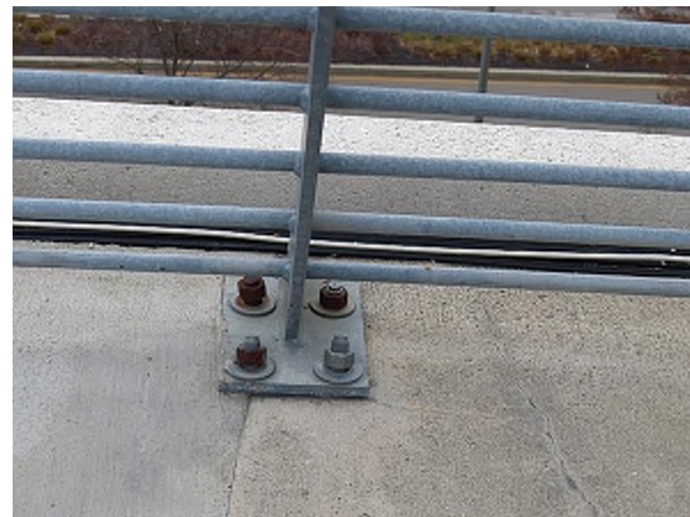
Bent threaded rods and rusted rods and nuts at the handrail attachment for the pedestrian bridge leading to the party deck
