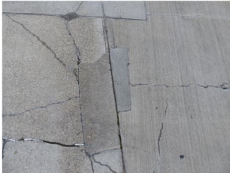
Cracking along a previous concrete patch with failed sealant along one crack (Upper Concourse, west)
