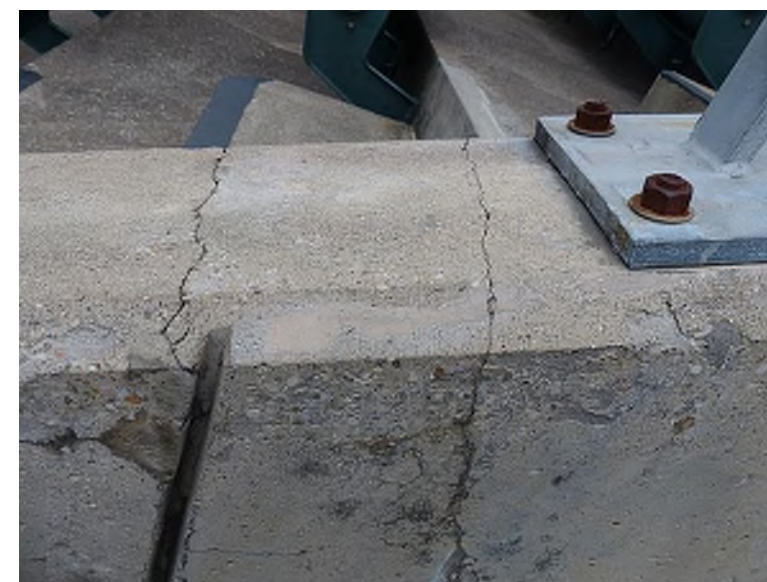
Concrete cracking along the top of the vomitory wall (South Seating Bowl, Section 154)
