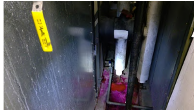
Chilled water leak at AHU-S-2 coil connection
