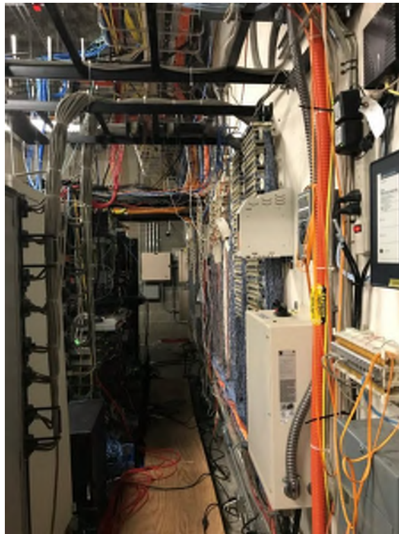
Wall mounted building copper infrastructure for the 700 building phone drops
