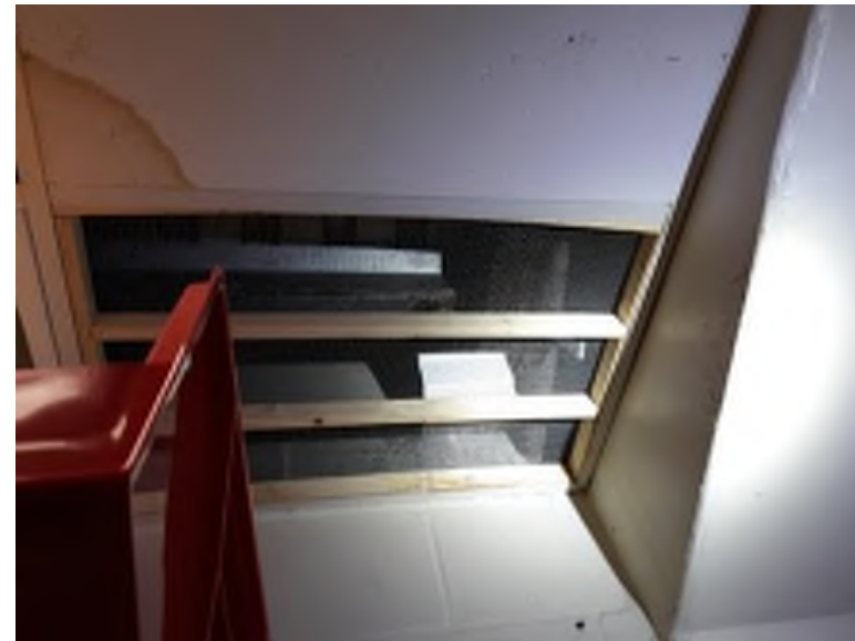
Wood frame with screen mesh. Note stain on ceiling tile.
