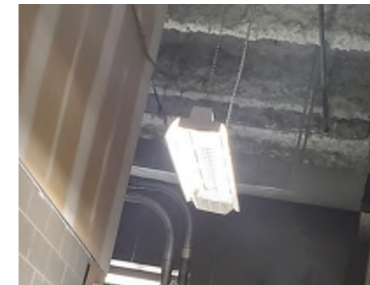
Typical mechanical/electrical area lighting
