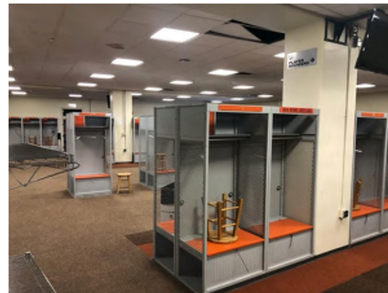
Visiting Team Locker Room with water damaged ceiling
