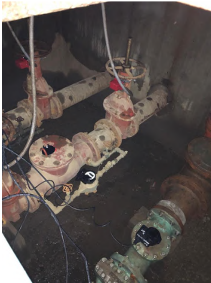
Fire pit remote meters & cables
