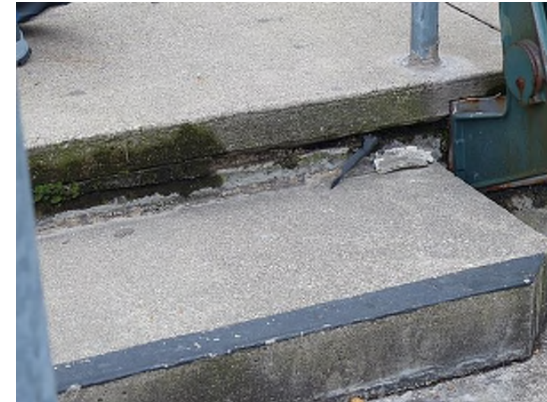
Deteriorated and missing sealant between the top precast riser beam and topping slab (South Seating Bowl, Section 158)
