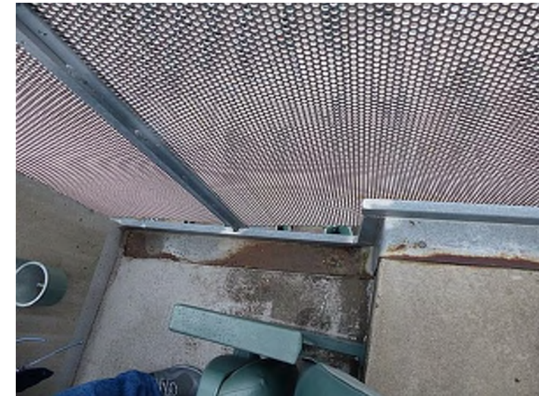
Corroded edge metal along end raker beam (Club Level)
