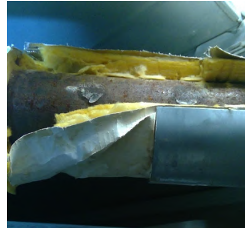
Pipe corrosion due to missing insulation and vapor barrier
