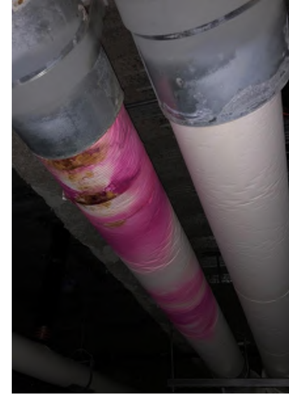
Leak in the dual temp main in Mezzanine Sector 8. Rust coloring of insulation indicates possible pipe corrosion under insulation.
