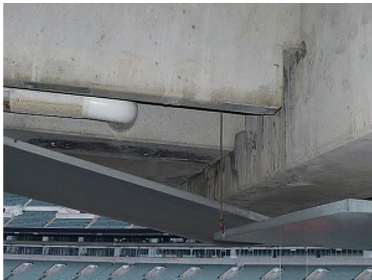
Staining and efflorescence on precast concrete members in the location of water leak locations above metal pans used to collect the leaking water (Plaza Level, north end of east concourse)
