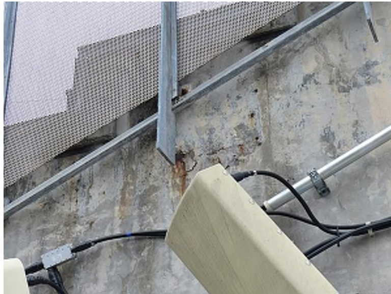
Delamination and corrosion along the exposed side of the raker beam (Club Level, south end of east seating bowl)
