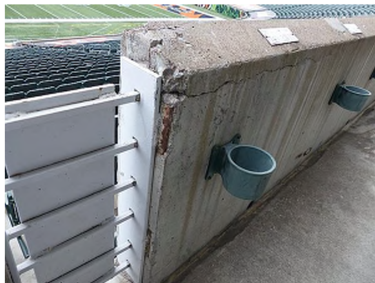
Cracked and spalled concrete located at the embedment plate of the railing wall (Lower Bowl, Section 140 Row 32W Seat 11)
