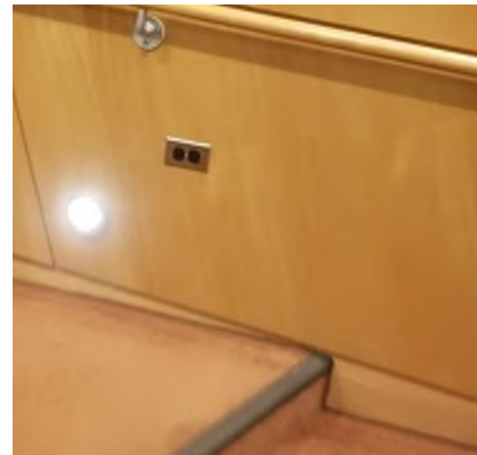
Auditorium step lights
