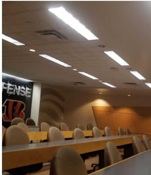
Small Auditorium lighting
