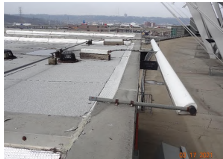
Light fixture attachment at concession area
