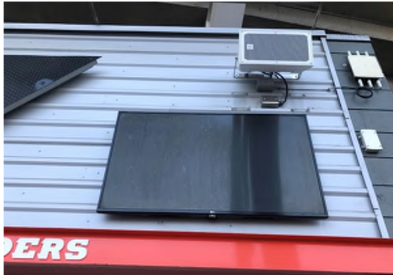
Access point next to speaker on concession stand fascia
