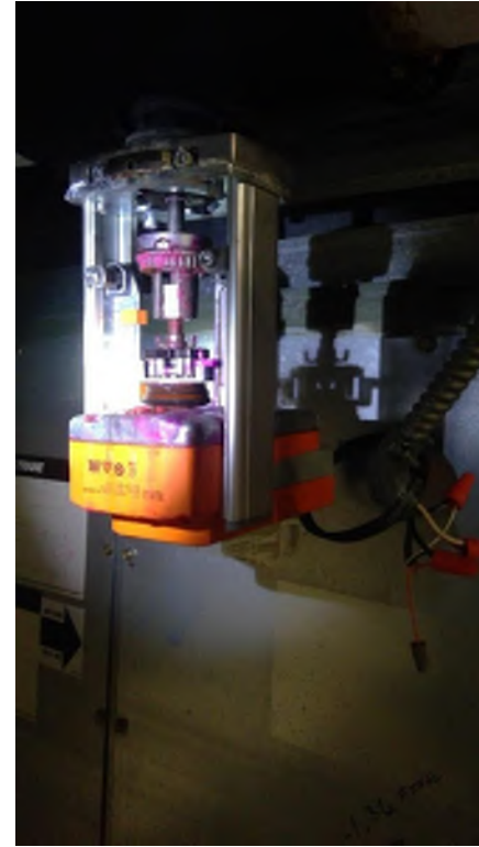
Major leak from control valve of AHU-UL-8
