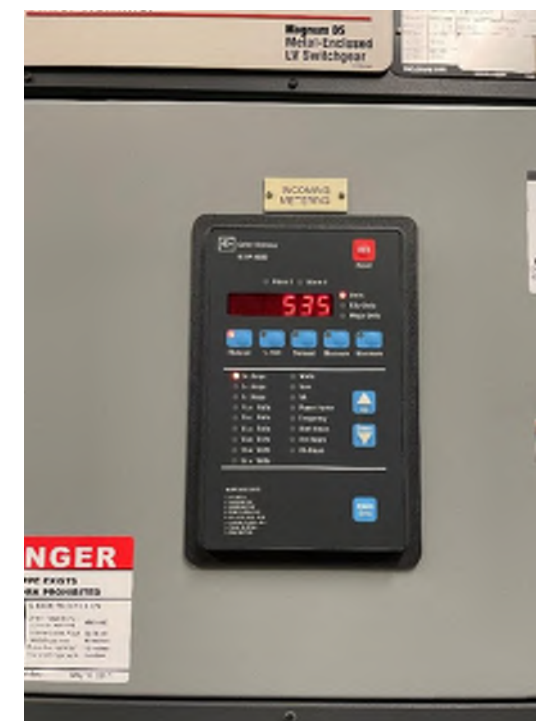
Typical substation main meter
