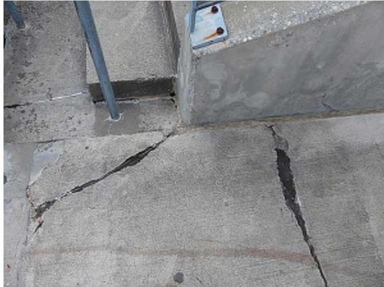
Deteriorated sealant used for repair in topping slab adjacent to a vomitorium (South Seating Bowl, Section 152)
