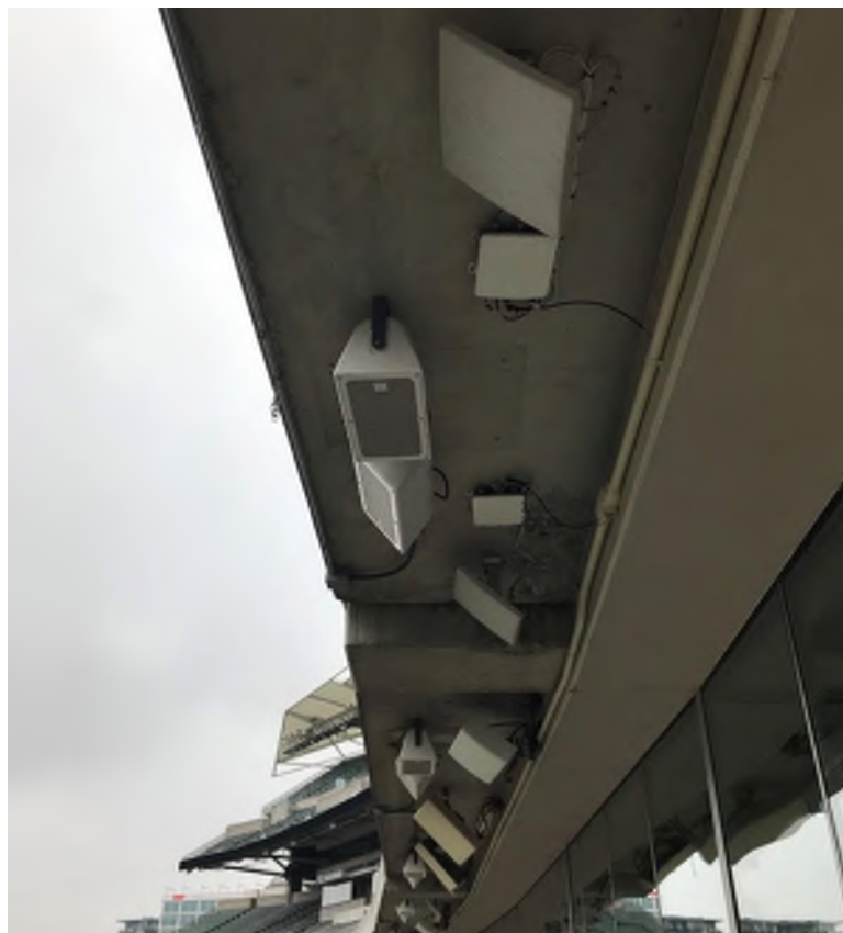
Access points and panel antennas on the bowl fascia precast
