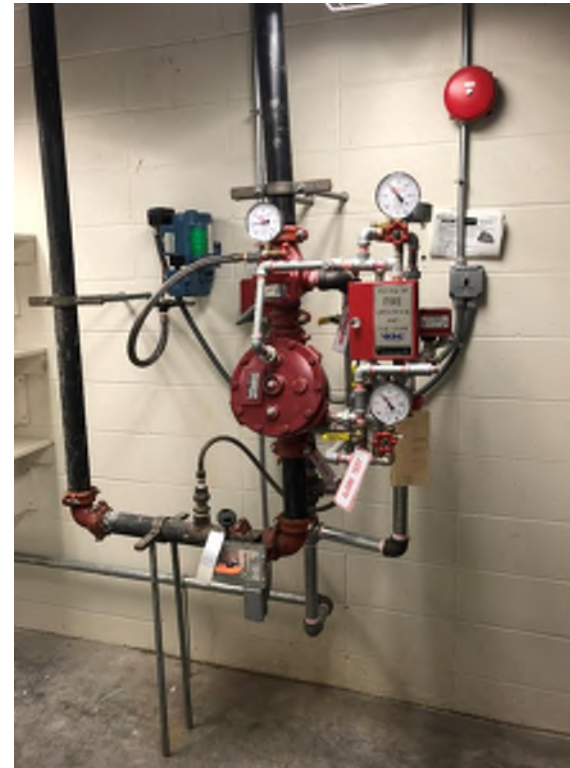
Pre-Action System & Air Compressor
