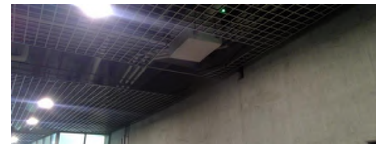
Suspended grease interceptor
