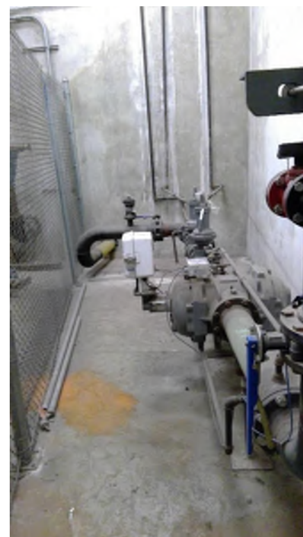
Natural gas entry into building
