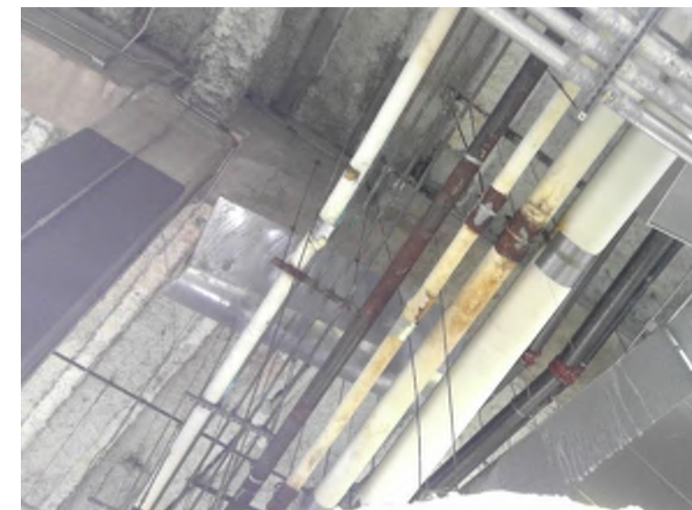
Natural gas pipeline corrosion due to water leakage onto pipe exterior. Damage to other exposed metal is evident, indicating external sources of water onto the pipe. Another indication of an external source is the white streaking down the duct shown in the lower right of the image.
