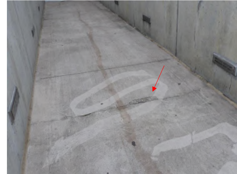
Crack and spall located in the topping slab of the vomitorium (South Seating Bowl, Section 152)
