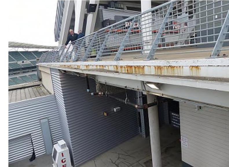
Corrosion residue along slab edge where water drains into the attached gutter (Club Level, north concourse)
