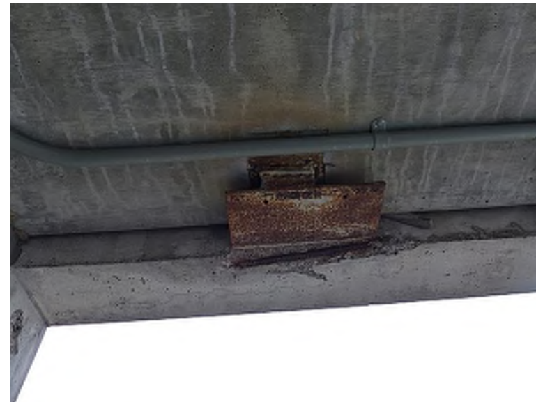
Corroded clip angle between precast slab and concrete beam (Upper Concourse)
