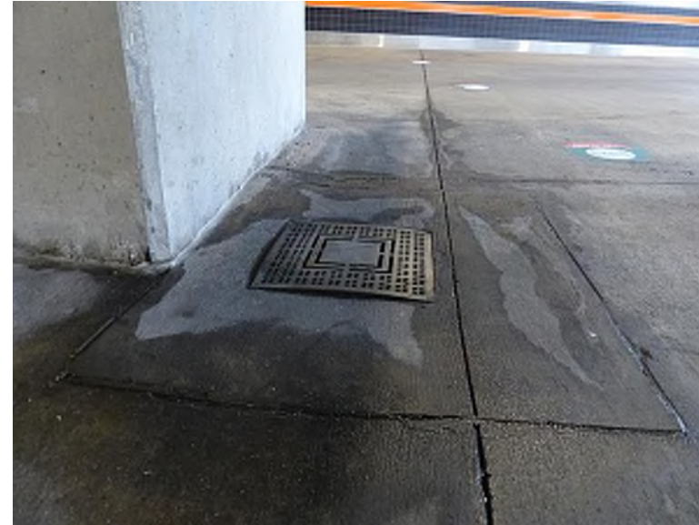
Buckled drain cover adjacent to concessions (Plaza Level, northeast concessions)
