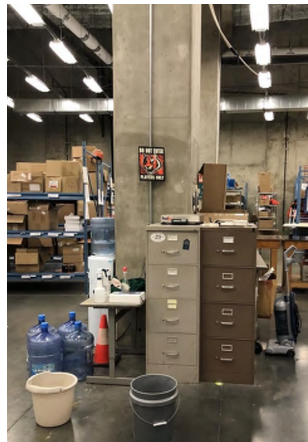
Retail Warehouse has water leaking from Plaza deck above
