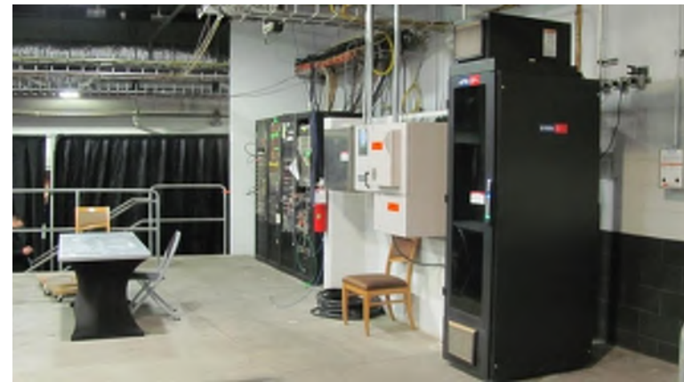
NFL Technology rack at truck dock (nearest rack)
