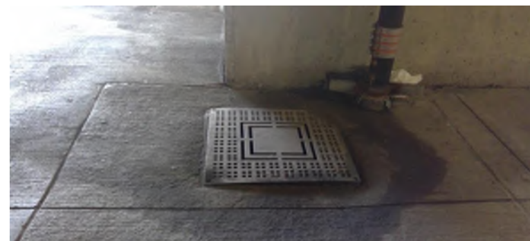
Bulged concourse drain cover
