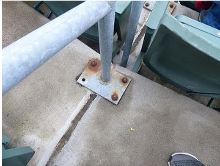
Corroded railing fasteners with one bolt missing (Club Level, Section 202)
