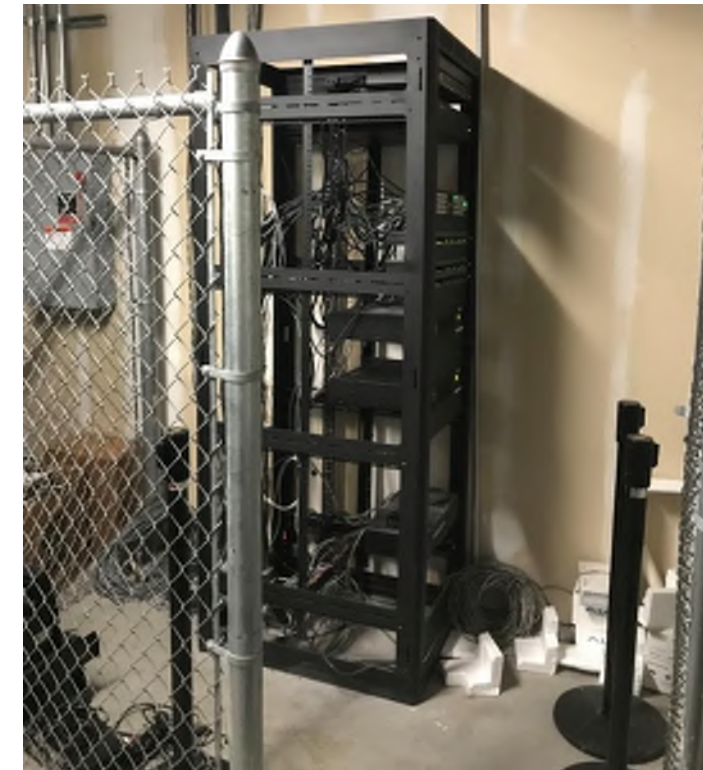
Club sound system rack in local Amp room
