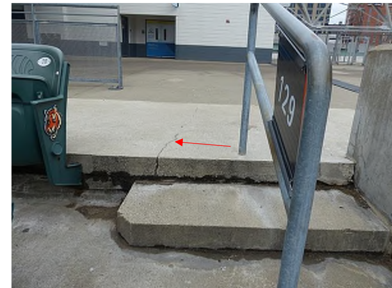
Crack in topping slab extending through the slab edge (Plaza Level and Lower Bowl, Section 129)
