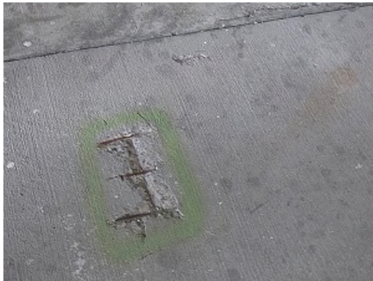
Exposed mesh in architectural topping slab at the plaza level (Upper Level Suites, west at south end)
