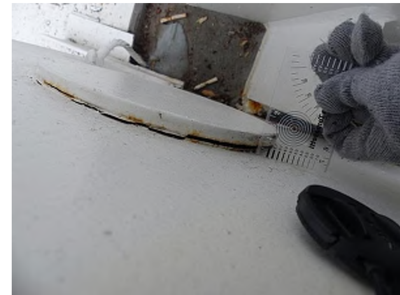
Gap present along steel pin end cap and upstand plates that receive the boomerang column (Club Level, north concourse)
