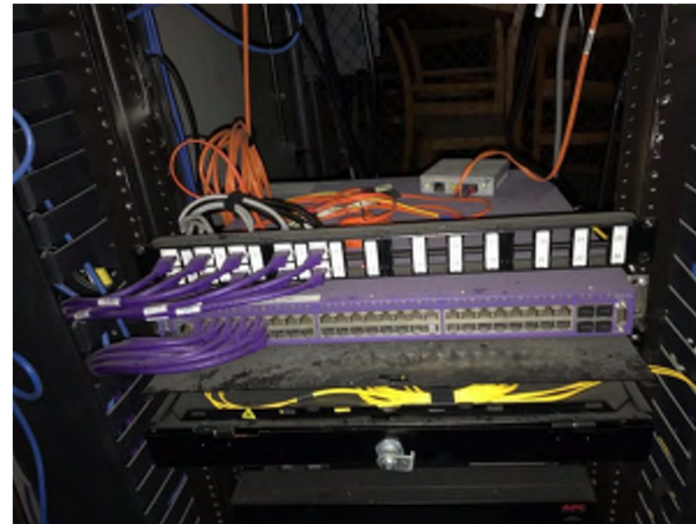
Extreme Networks switch connecting access points
