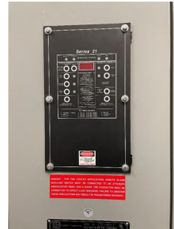
Non-functioning substation transformer cooling controls
