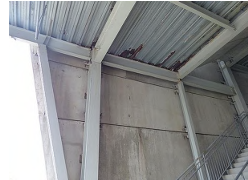
Corroded metal decking located beneath a stair landing above the plaza concourse (Club Level, southwest stairs); steel correction and re-coating is an ongoing, yearly capital project at PBS
