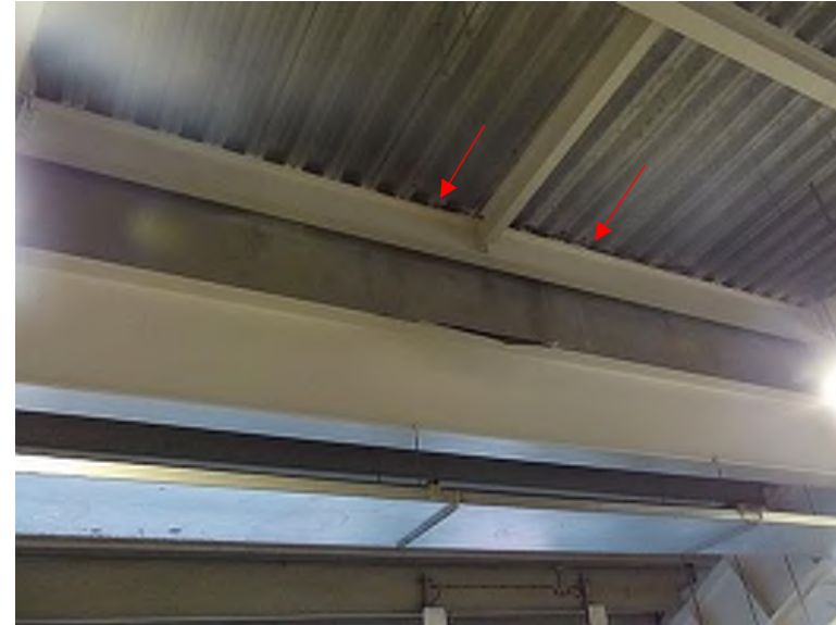
Corroded metal decking and staining on metal framing above metal pans used to collect leaking water (Plaza Level, north end of east concourse). Note that owner has begun metal decking replacement at stairs and ramps during 2021.
