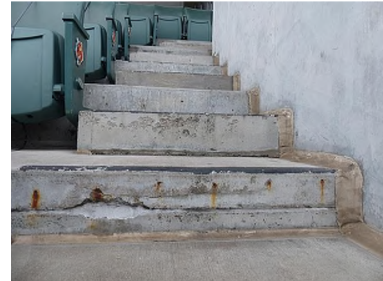
Exposed transverse reinforcing steel along the vertical surface of a precast seating riser (Club Level, Section 202 Row 14)
