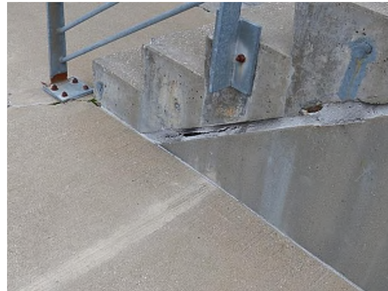
Deteriorated sealant between the precast vomitory walls and steps (North Seating Bowl, Section 226)
