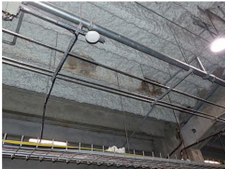
Delaminated acoustic insulation on the underside of precast seating risers (Service Level, adjacent to column line 15)
