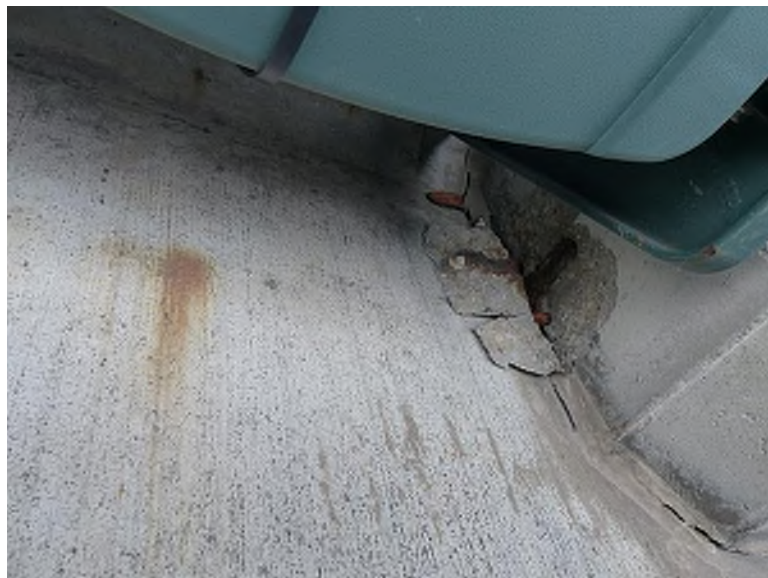
Delaminated concrete with exposed corroded rebar on the edge of the intermediate step (Club Level, Section 241 Row 14)
