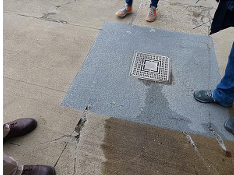
Failed concrete patches adjacent to the traffic coating along the floor drain (Upper Concourse, west)
