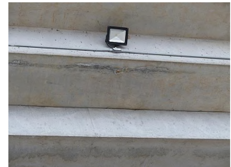
Leaching along the underside of the bottom tier of the precast concrete riser (Upper Concourse, east)
