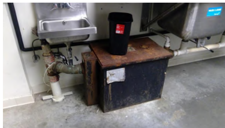
Floor mounted grease interceptor
