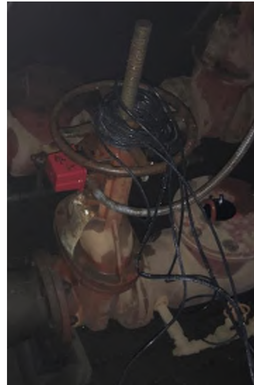
Fire pit remote meters & cables
