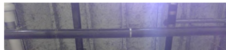
Uncorroded natural gas pipe.
