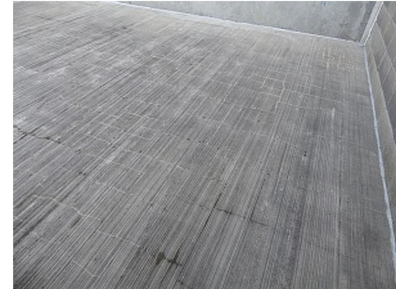
Cracked and deteriorated traffic coating at the upper concourse level
