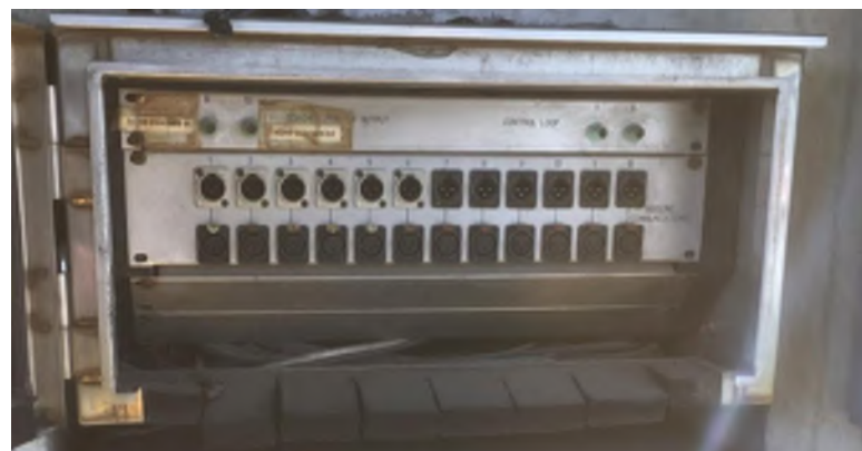
Old analog coaching cabling at visitor field sideline
