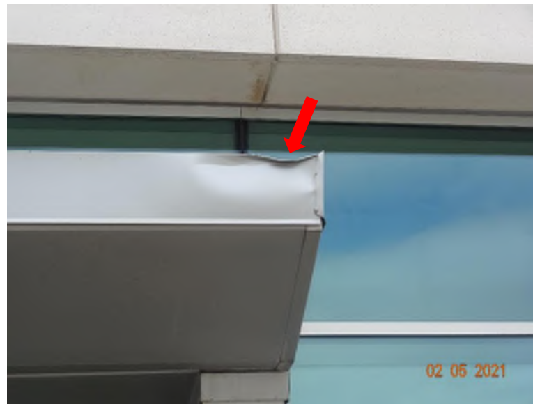
Pro Shop canopy – dented corner
