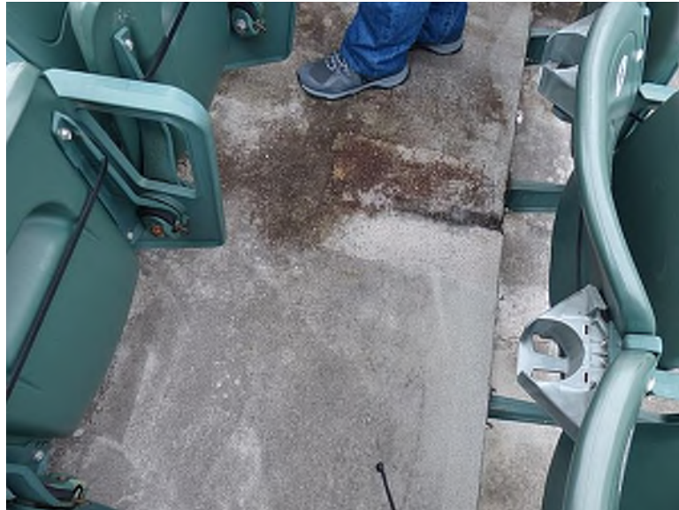
Deteriorated traffic coating along expansion joint (South Seating Bowl, Section 158)
