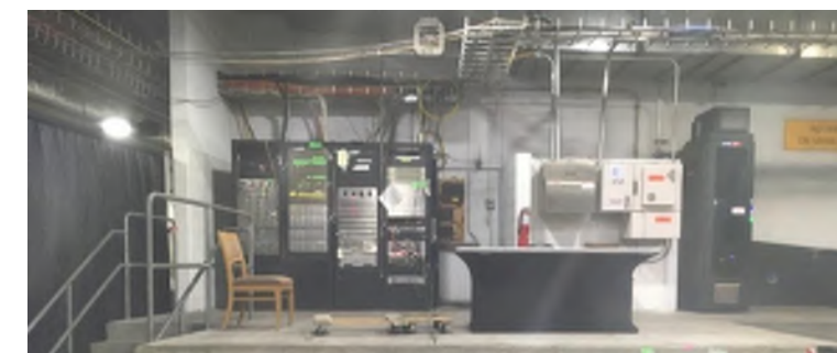
Existing network racks, AT&T (common carrier), and NFL Technology racks
