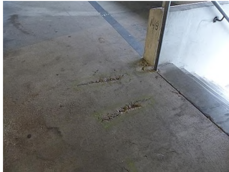
Exposed mesh in structural topping slab at the plaza level (Plaza Level, Section 148)
