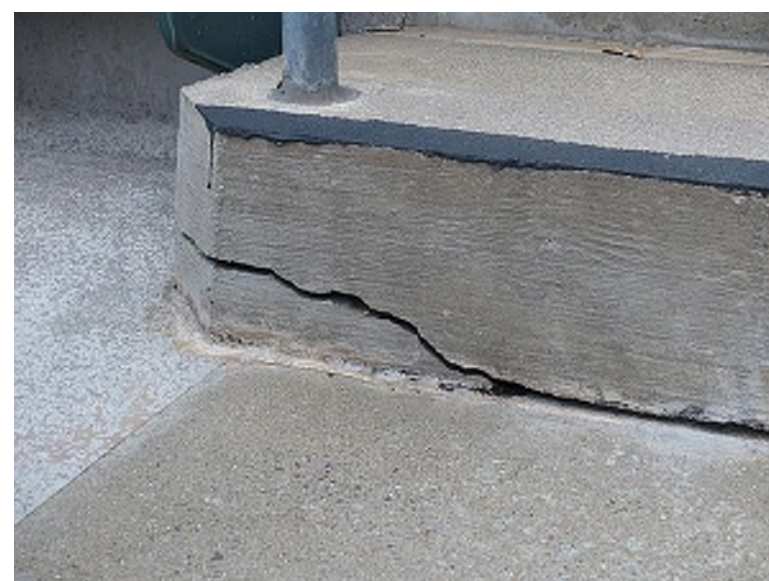
Cracking at the bottom corner of the intermediate step at the location of the stanchion (North Seating Bowl, Section 228 Row 8); sealants should be installed to prevent "freeze/thaw" issues from occurring
