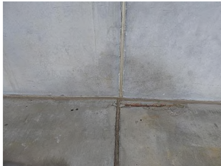
Exposed mesh in precast slab adjacent to plaza suites (Plaza Level, Section 136)
