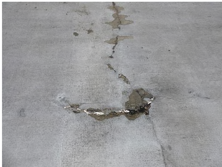
Failed concrete patch beneath deteriorated traffic coating (Club Level, north concourse)
