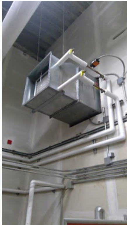
Fan Coil Unit STX-US-1 inside the East boiler room
