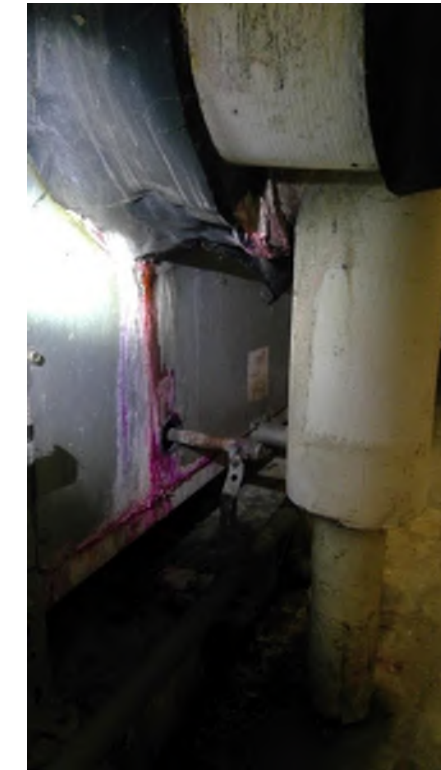
Leak at coil connection of AHU-P-1
