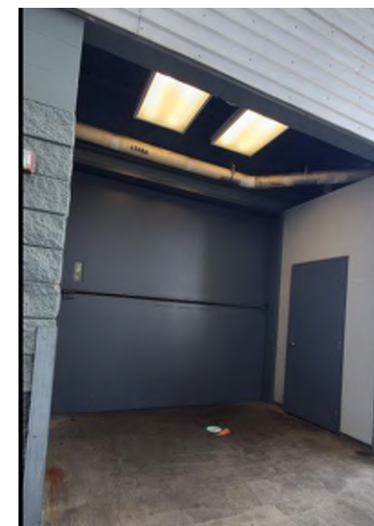
Service area entrance light
