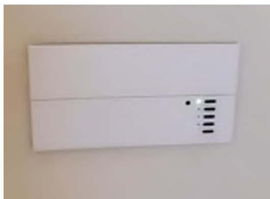
Club Suite lighting controls, typical
