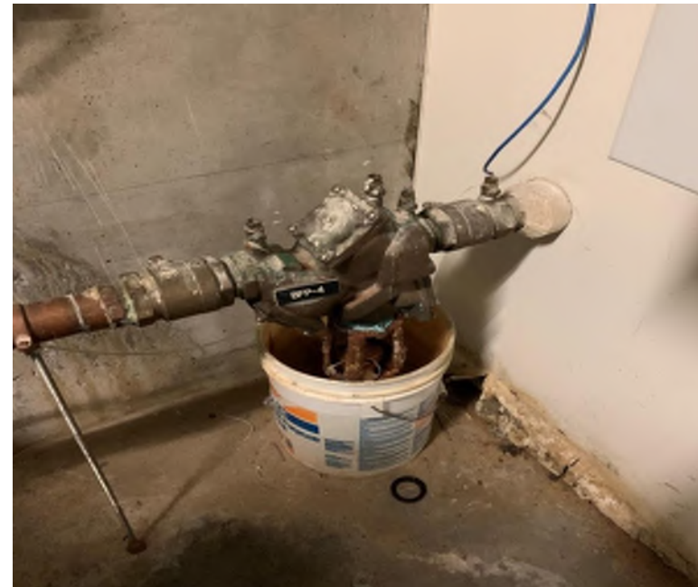
Irrigation backflow preventer
