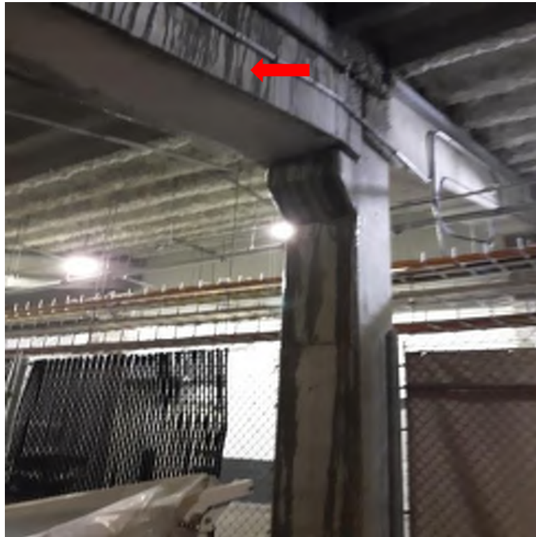
Interior moisture damage – moisture on beam
