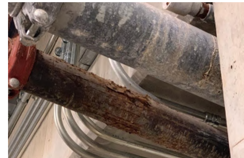
Rusted steel piping (Fire Line)
