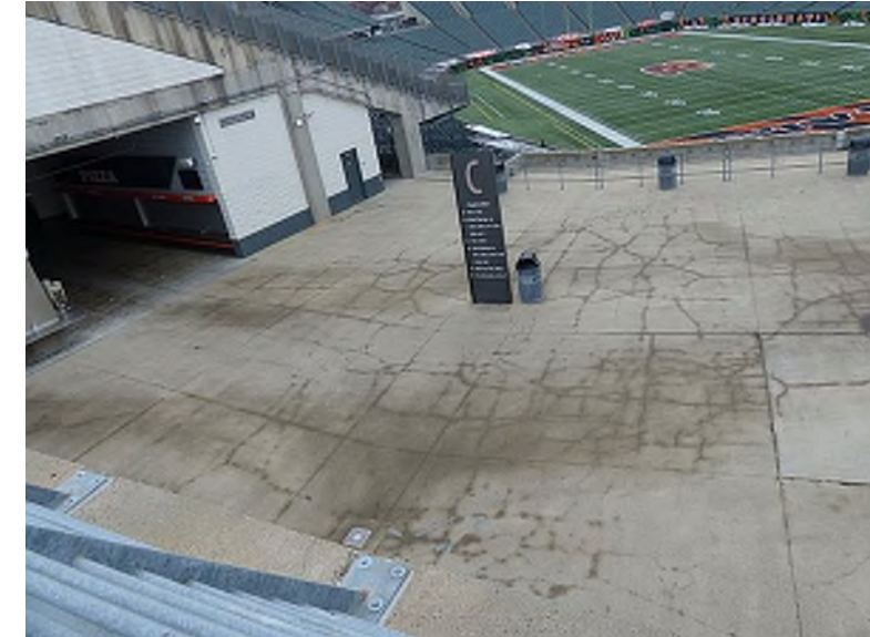
Extensive cracking throughout topping slab (Plaza Level, northeast concourse)
