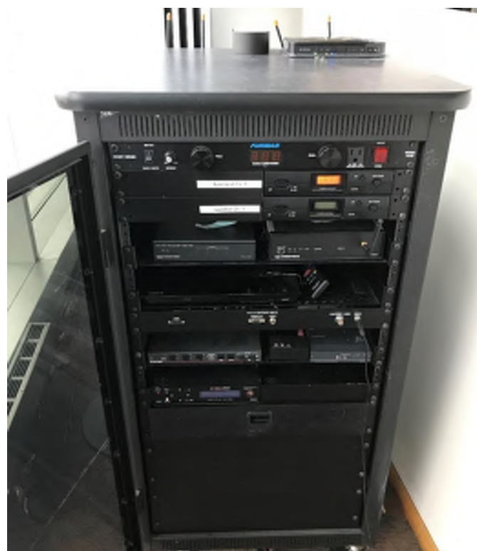
Local source input rack behind the bar
