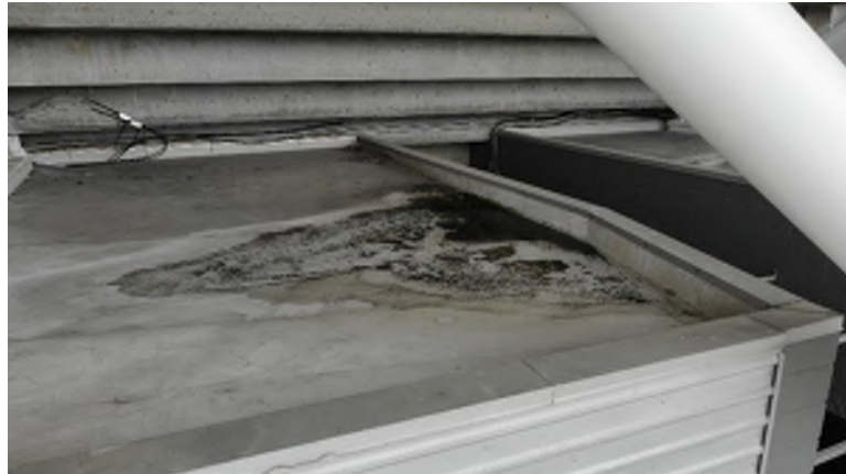
Ponding water on EP membrane
