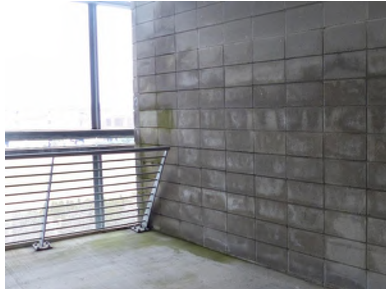
Biological growth located on the CMU wall along the landing on the ramp (northwest ramp)
