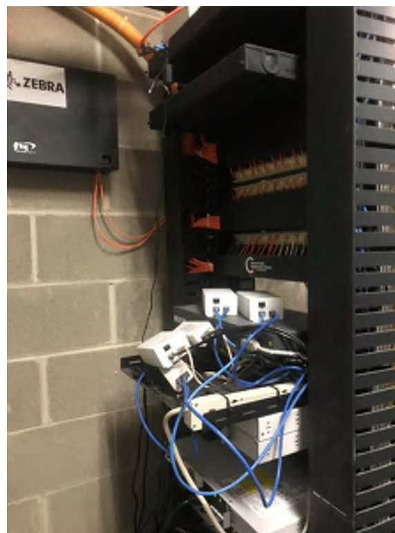
Security camera power injectors
