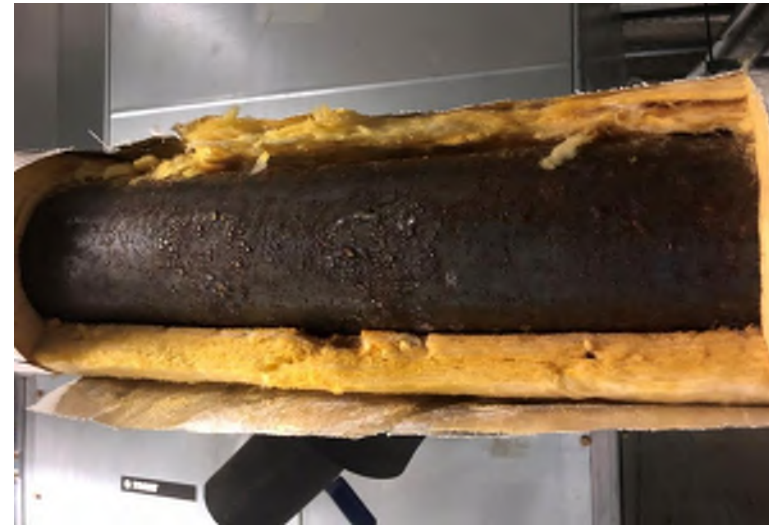
Pipe corrosion due to missing insulation and vapor barrier. Water is condensing out of the air onto the pipe. Water will cause corrosion of the pipe over time.
