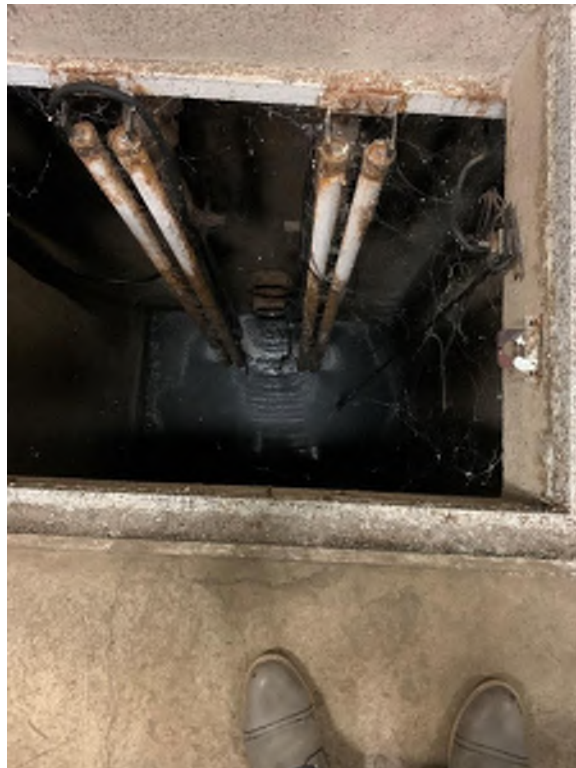
Rusted sewage pump rails
