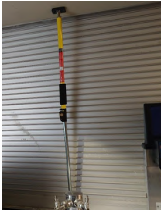
Jack at overhead door
