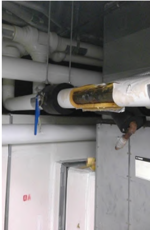
Butterfly valve almost completely closed to reduce flow through AHU-UL-6.
