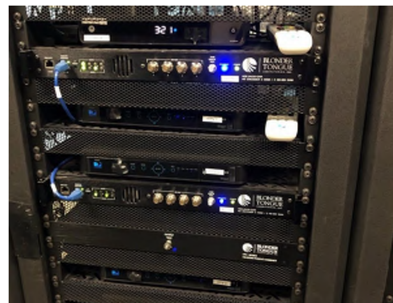
Satellite receivers & in-house feed encoders
