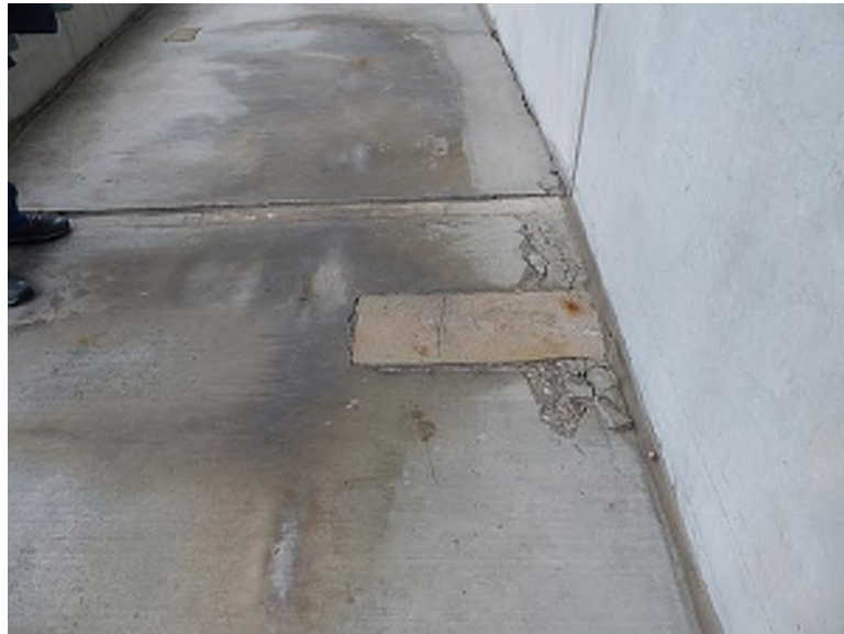
Spalling adjacent to a previous repair in the topping slab along plaza level suites (Plaza Level, Section 140)
