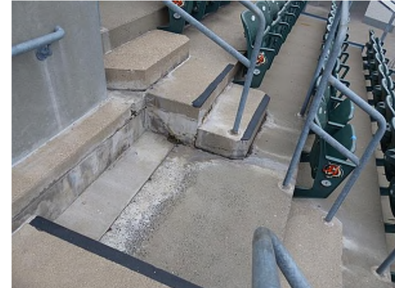
Water leaking beneath steps at north end of stadium (North Seating Bowl, Section 230 Row 10)
