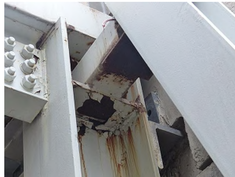
Corroded ramp structural steel (southeast ramp); steel correction and re-coating is an ongoing, yearly capital project at PBS
