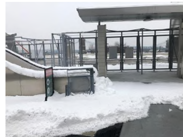
Gate E and Escalator: Inadequate clearance inside gate. No wayfinding present.
