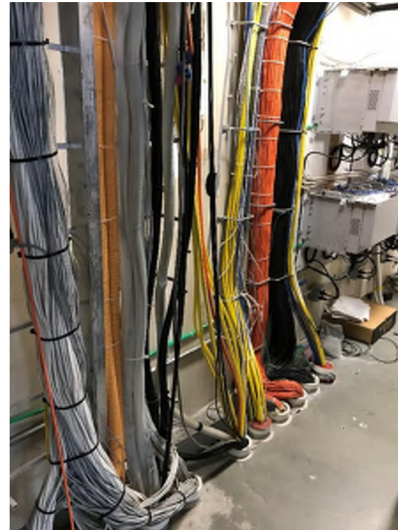
Press level IDF floor penetrations all full beyond industry recommended capacity
