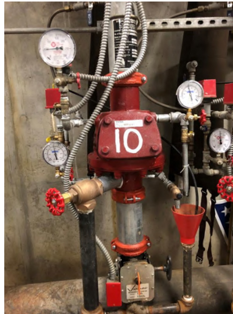
Replacement dry valve with new gauges and trim.
