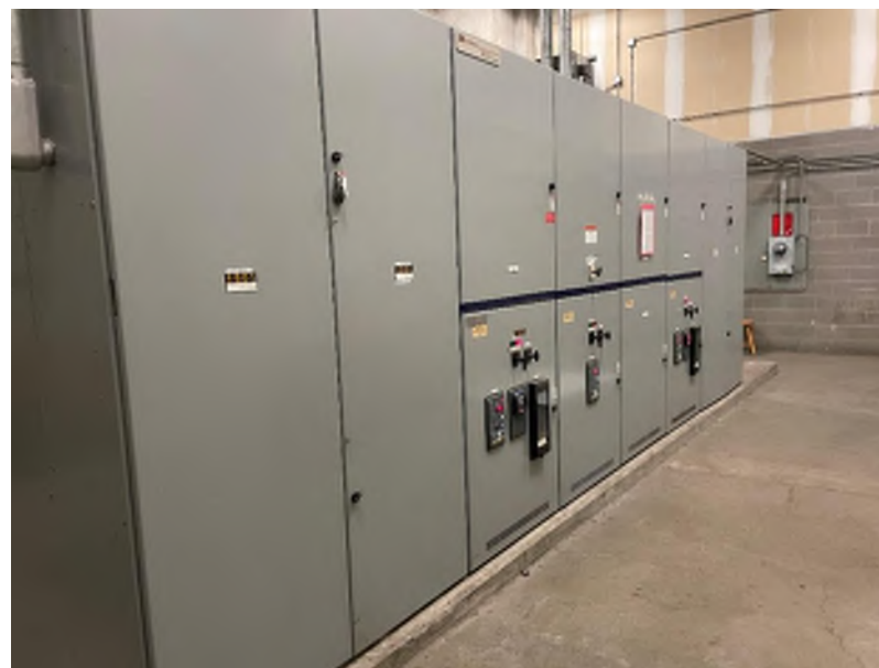
Medium-voltage service entrance main-tie-main and metering
