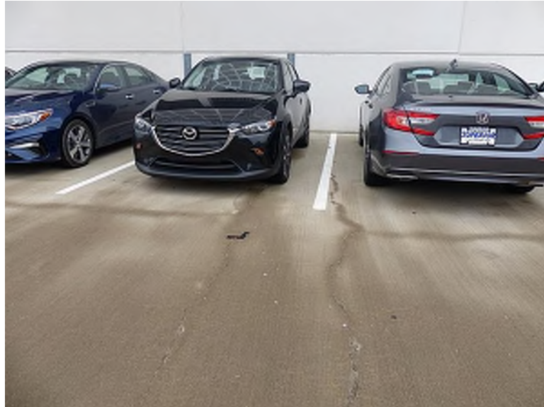
Cracking in parking lot topping slab that follows edge of concrete beam below
