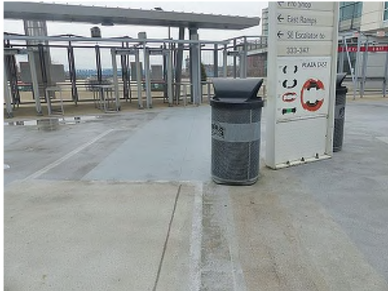
Multiple patches of traffic coating present with a crack in the coating along the construction joint (Plaza Level, south concourse); coating is scheduled to be replaced in 2022 at this location and the south end zone in general
