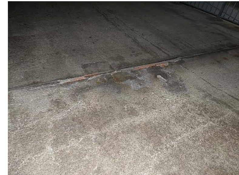
Cracked and deteriorated traffic coating at the plaza concourse level
