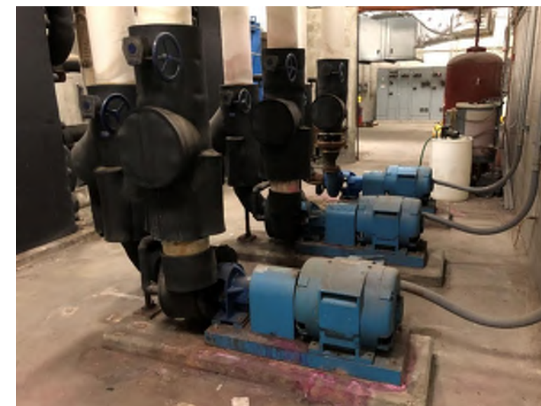
Stadium chilled water pumps with glycol residue from seal leakage
