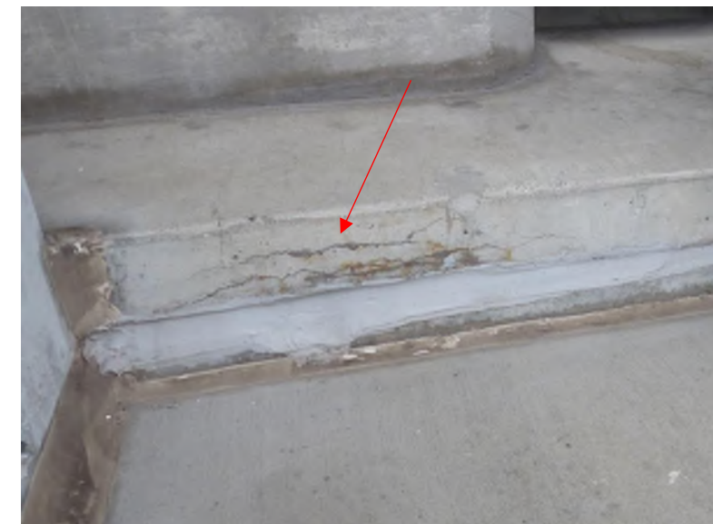
Concrete and corrosion delamination along edge of precast riser beam (Club Level, Section 202 Row 31)
