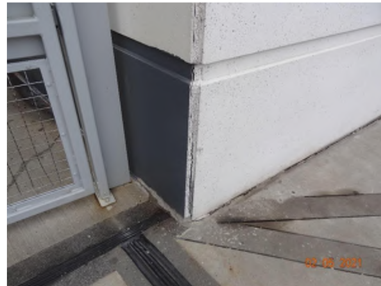
Precast concrete wall panels – sealant failure
