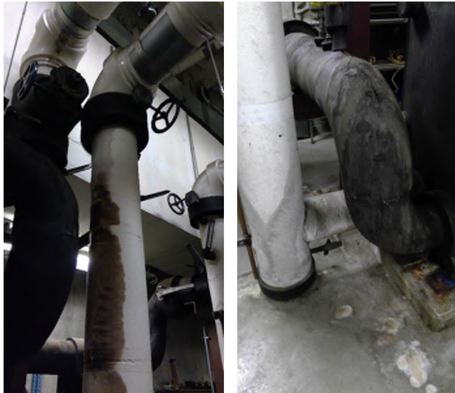
Pipe insulation mold and damage from water leakage at pipe flanges
