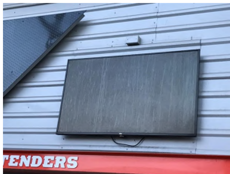
Fully exposed non-outdoor rated television
