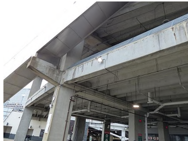
Multiple locations of exposed reinforcing steel along the length of a precast beam (Plaza Level, southeast concourse)
