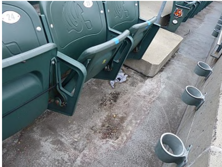
Deteriorated traffic coating on precast riser surface (North Seating Bowl, Section 126 Row 1)
