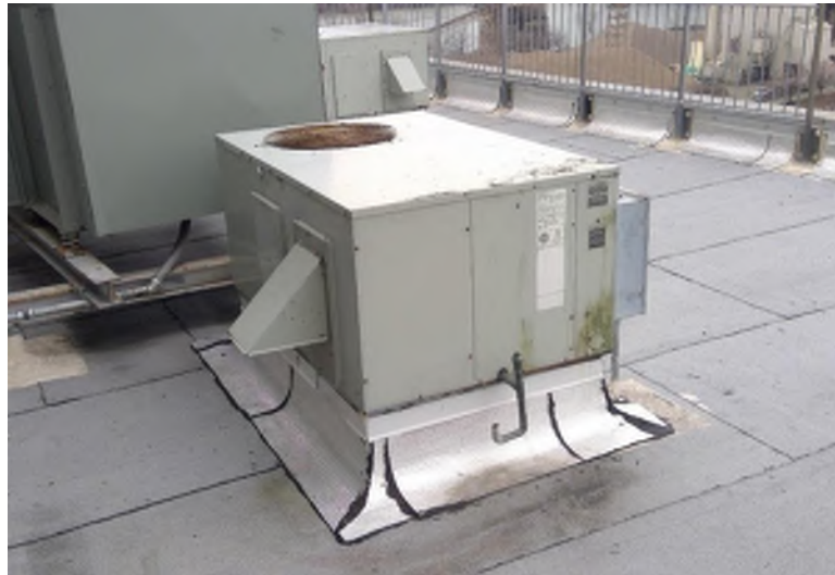
RTU on roof in upper concourse
