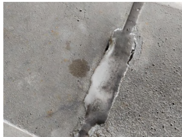
Exterior stair – failing joint sealant
