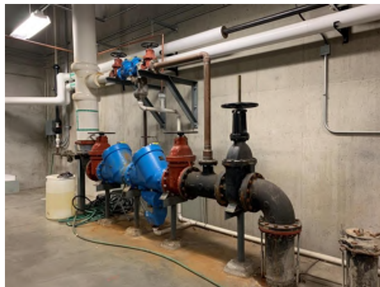
Building backflow preventer (Rebuilt in 2019)
