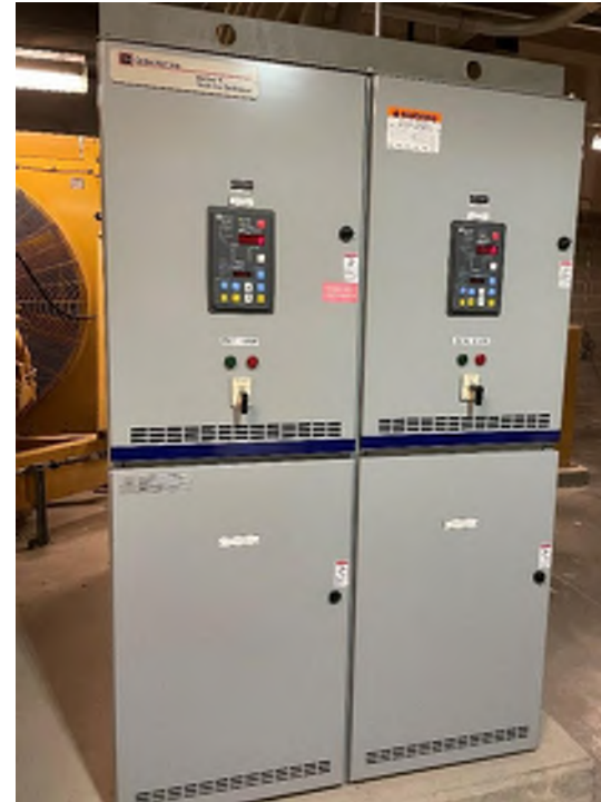
Generator distribution breakers to substations and fire pump
