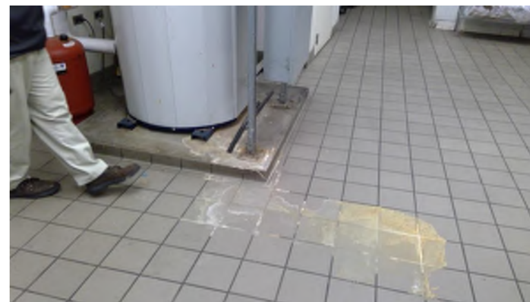
Main kitchen water heater
