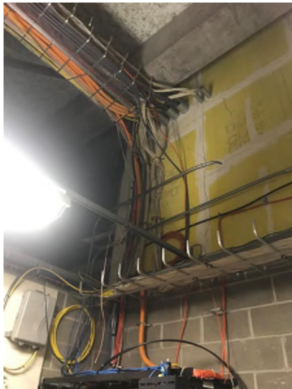
Upper cable tray and conduits in the IDF are full
