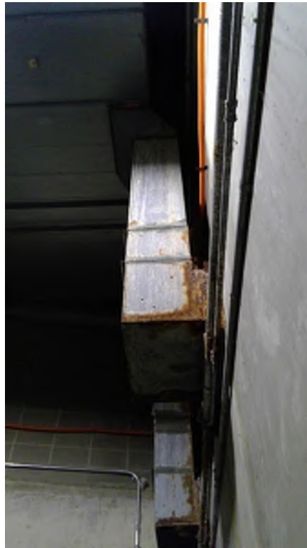
Corroded exhaust duct in sector 2 of the service level. Corrosion is external to the duct and close to areas with contact to the wall of the stadium.
