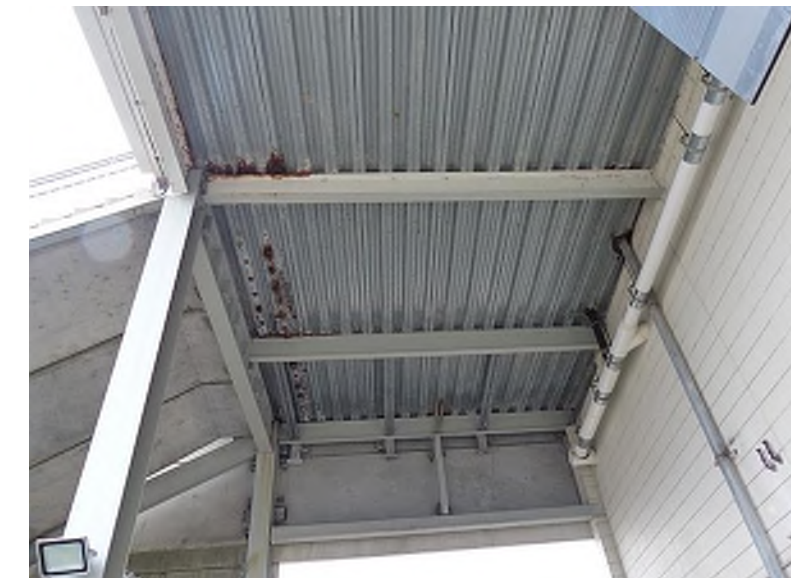
Corroded metal decking located on the underside of the upper concourse stair landing (southwest stairs, looking towards Upper Concourse); steel correction and re-coating is an ongoing, yearly capital project at PBS
