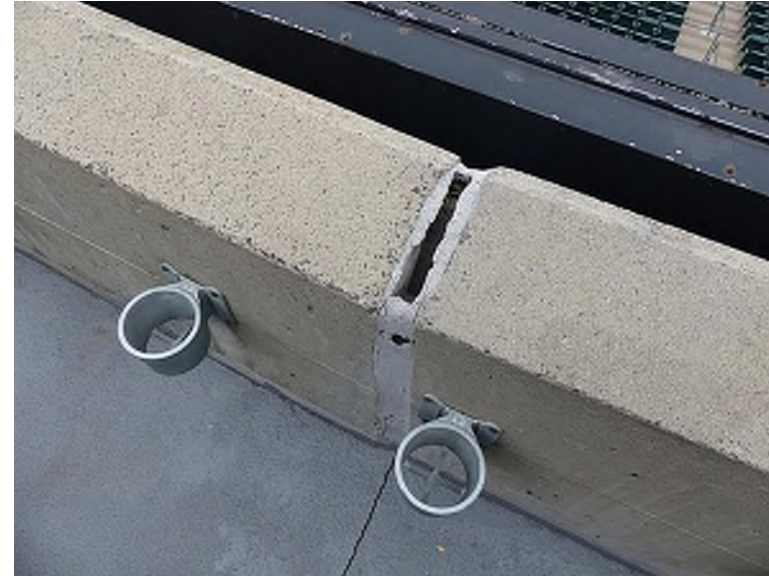
Sealant missing along the top portion of the railing wall (North Seating Bowl, Section 226), and is consistent throughout all vertical precast joints at all levels
