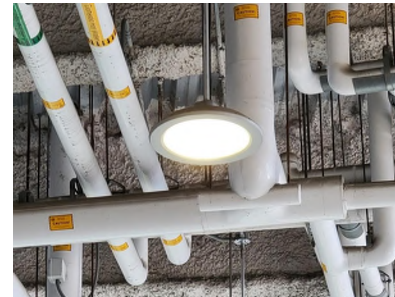
Typical Service Tunnel LED high bay lighting
