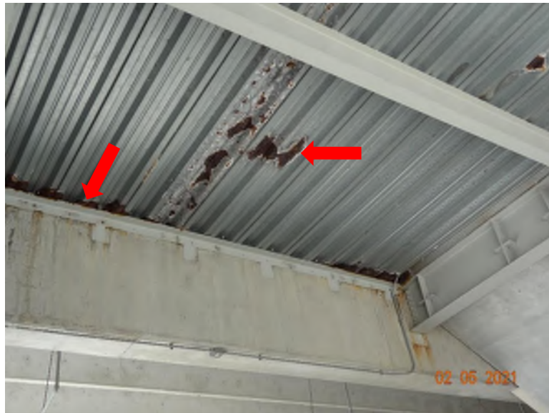
Exterior stair – rusting metal deck
