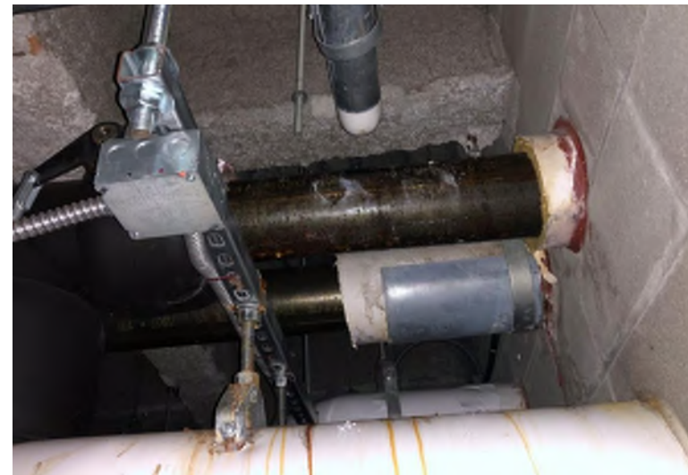
Exposed pipe in dual temp main in mezzanine in sector 5.
