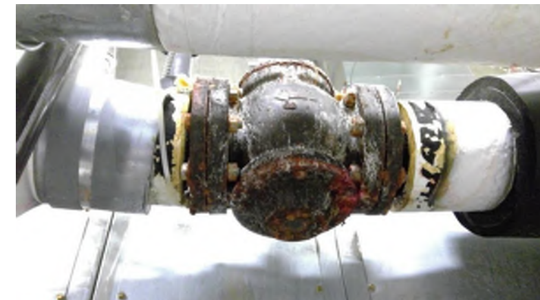
AHU-S-8 control valve corrosion.
