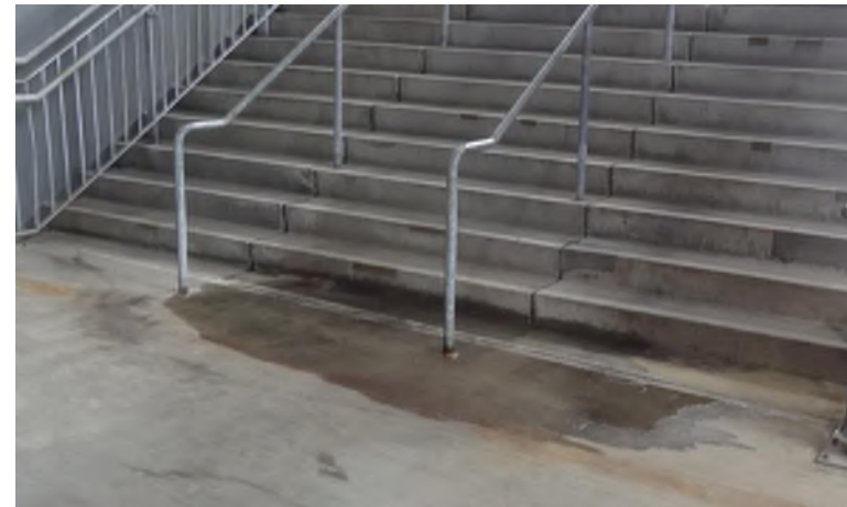
Exterior stair – ponding from leak above
