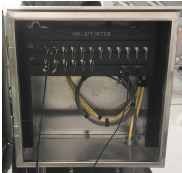
Example of permanent Motor Control Cabling
