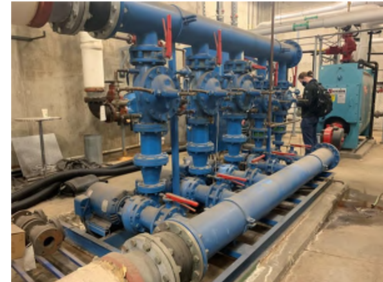
Domestic water pumps
