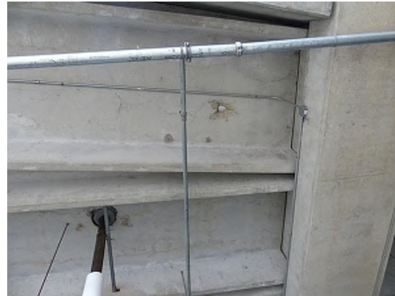
Localized concrete delamination on the underside of a precast double tee member (Club Level, northwest concourse)
