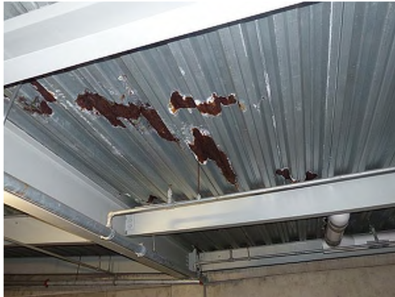
Corroded metal decking on the underside of the pedestrian ramp (near Field Level West)
