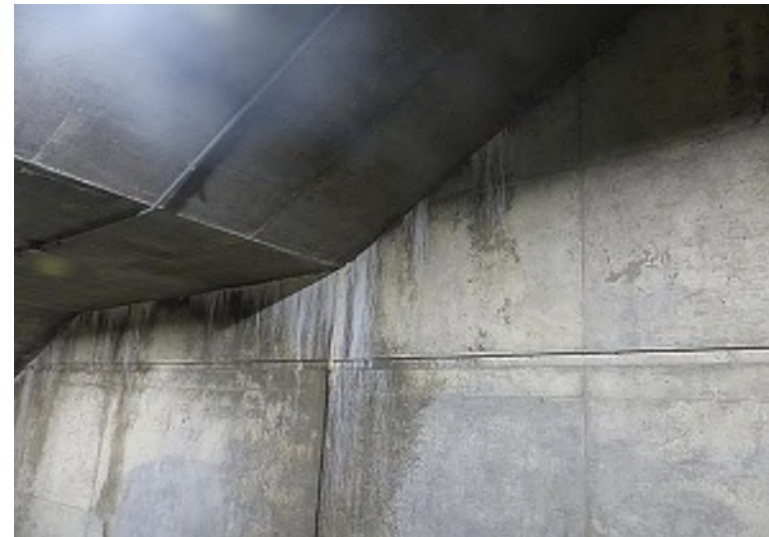
Concrete leaching below the exterior stairs that lead to parking on the east side of the stadium
