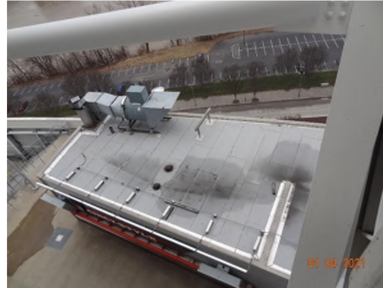
Equipment on roof
