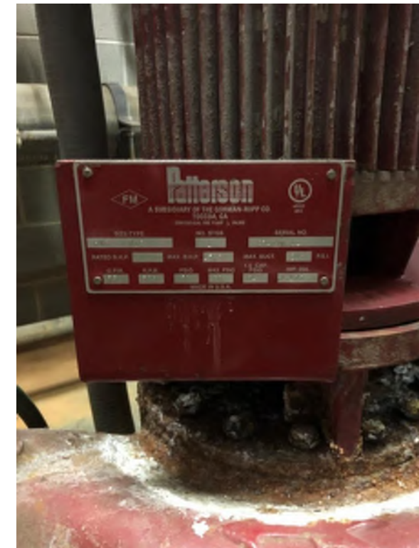
Fire Pump with repaired bad seal.
