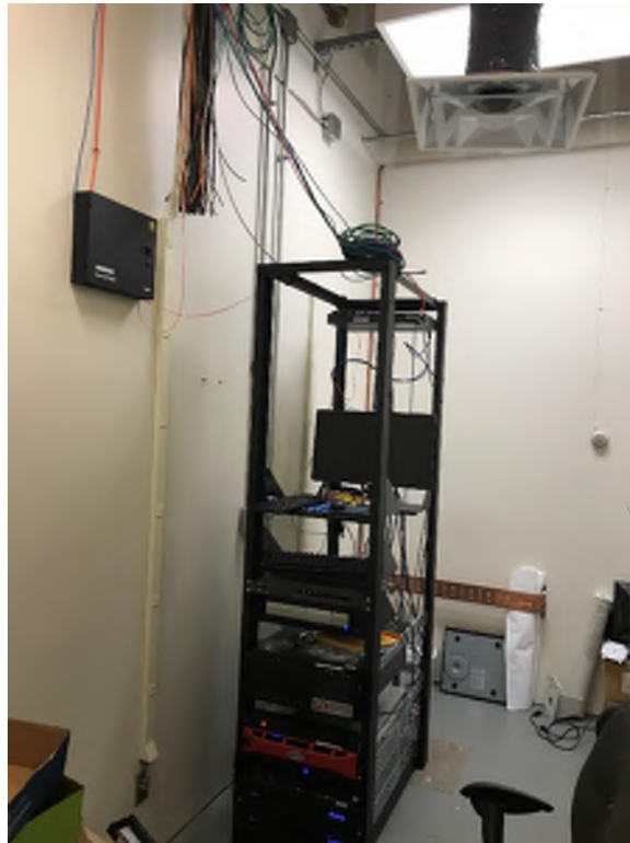
Security systems equipment rack and abandoned analog security camera cables
