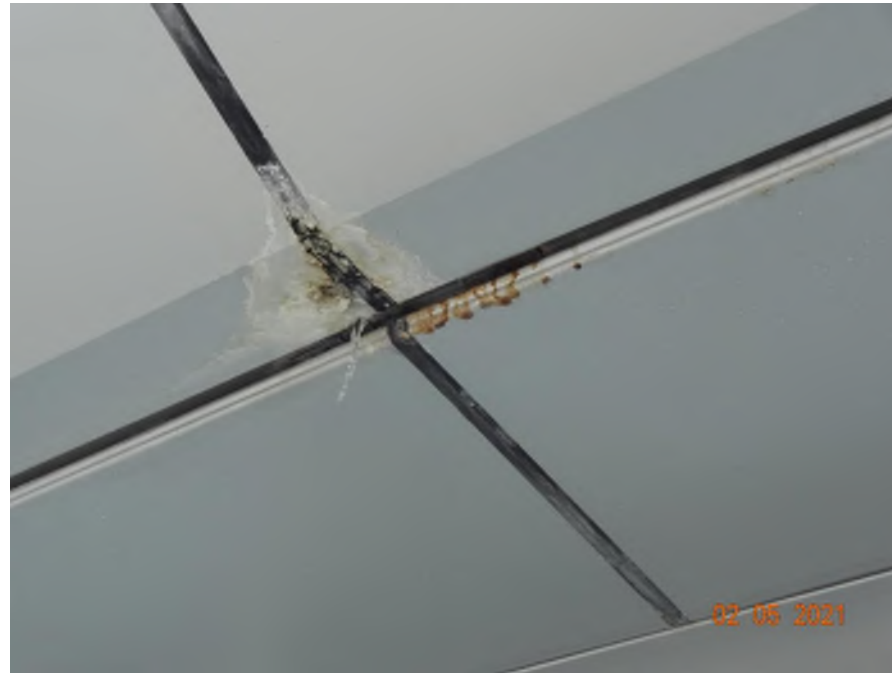
Pro shop canopy – soiling and deposits
