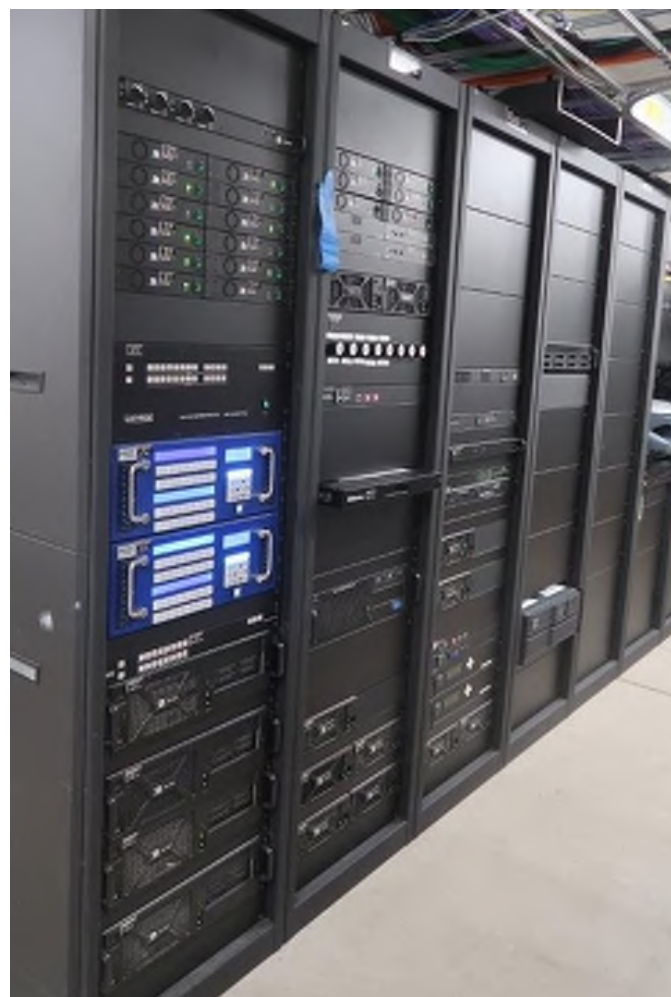
LED display control system
