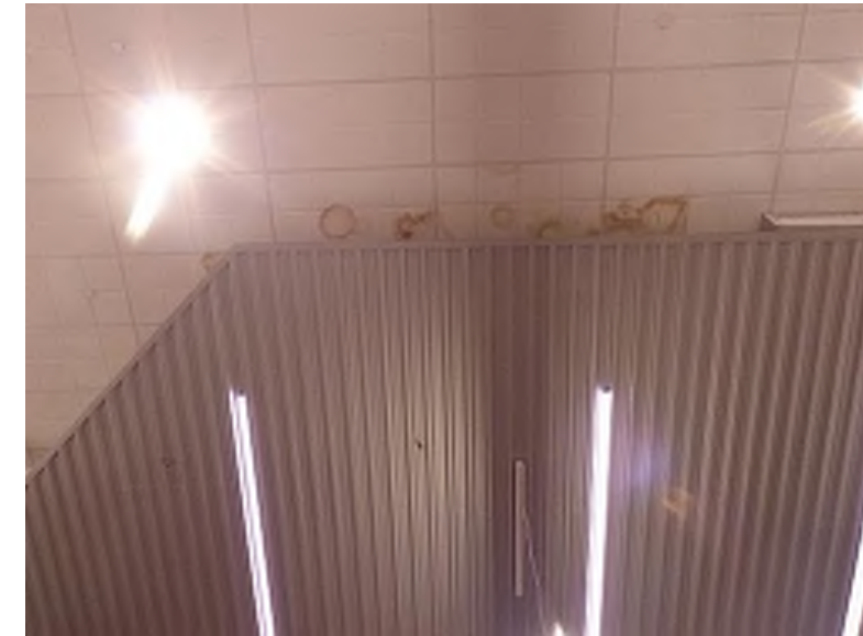
Water staining visible on ceiling tiles located in the fitness area, located below the plaza concourse
