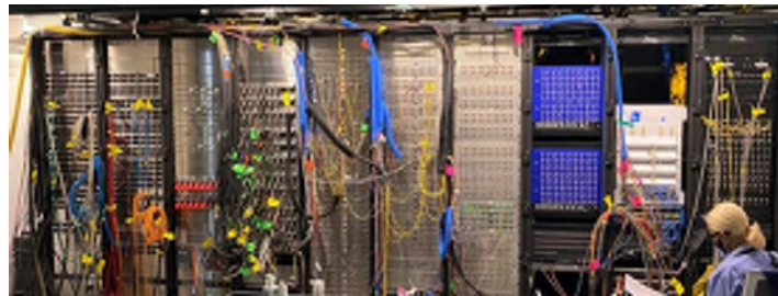
Cable termination room at SoFi stadium, for comparison of NFL Standards. Sliver panels are network installed, black/blue are in-house and common carrier I/O panels
