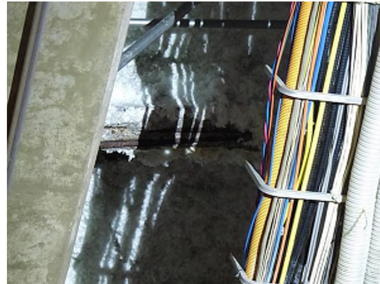
Delaminated acoustic insulation with exposed reinforcing steel on the underside of a precast seating riser (Service Level, adjacent to Vis Team Locker Room)
