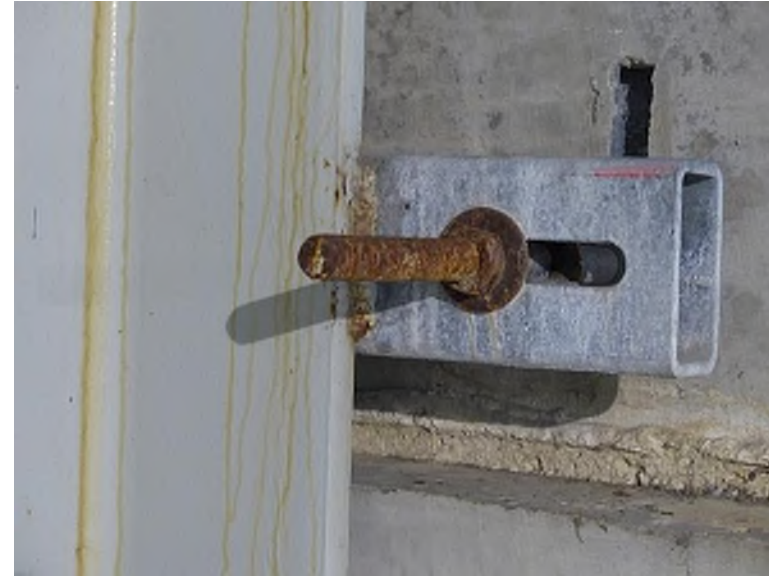
Corroded bolt, nut, and washer at the connection between the precast faced panel and steel support structure (Southeast Ramp)
