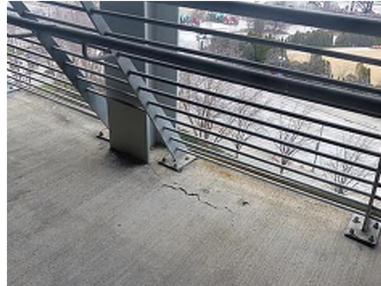
Delaminated concrete adjacent to the railing anchorage (northwest ramp)
