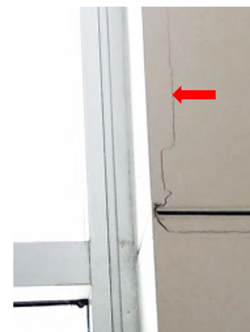
Cracking in gyp board next to curtainwall
