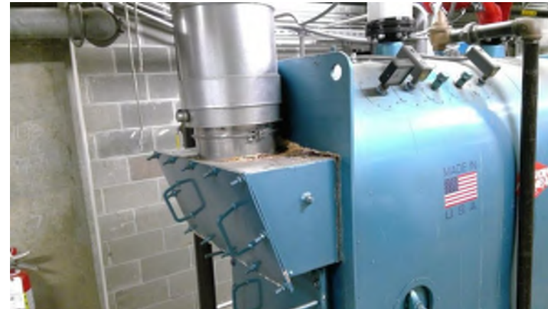
Corrosion to boiler and flue from water accumulation
