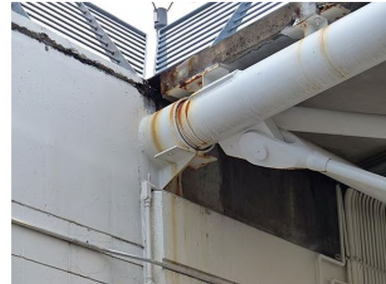
Deteriorated concrete and rusted steel where the bridge terminates
