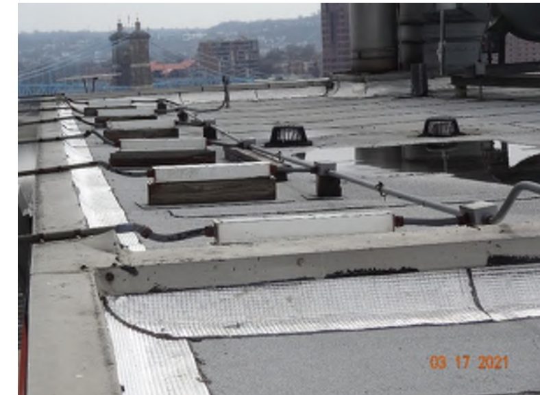
Wood blocking supports for electrical conduit on roof
