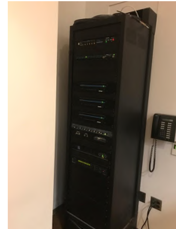
Team theatre equipment rack
