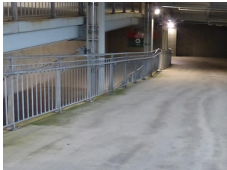
Biological growth along the edge of the pedestrian ramp (southeast ramp)
