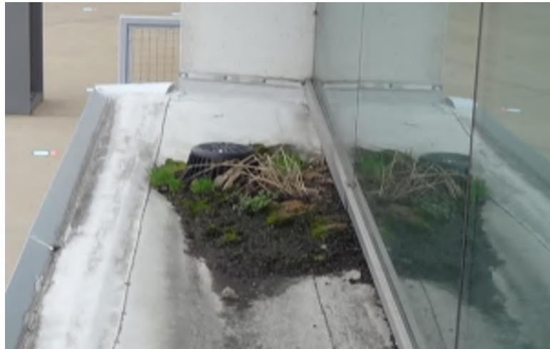
Biological growth at pro shop roof drain
