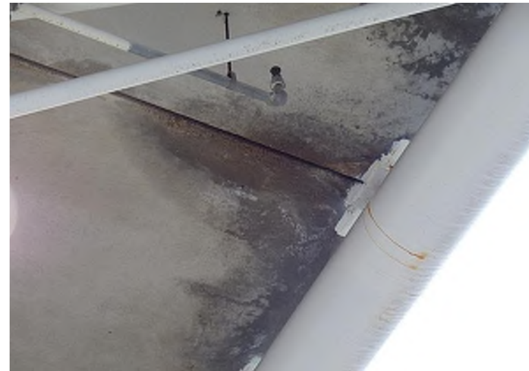
Efflorescence on the underside of the pedestrian bridge precast concrete plants
