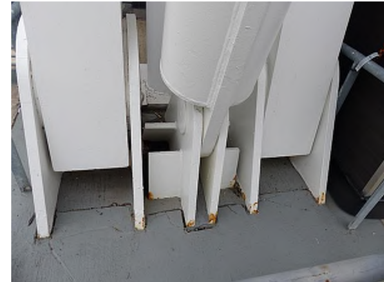
Corrosion present at the interface between the steel boomerang column base and concrete topping; boomerang steel was painted in 2019.
